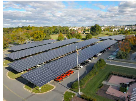
Microgrid at the Public Safety Headquarters
