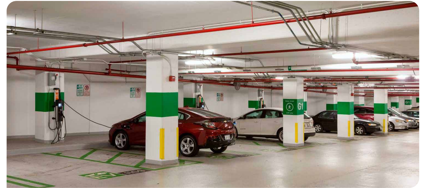
Private electric vehicle being charged at a County parking garage
