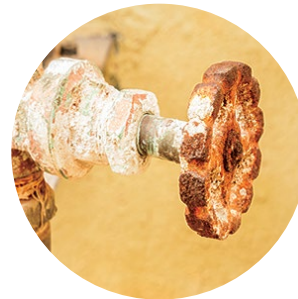
CHLORIDE corrosion, salty taste
