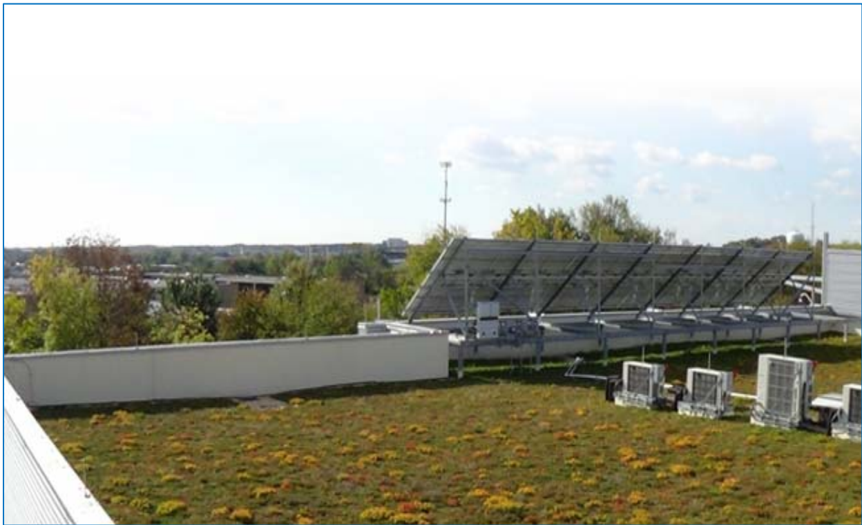
Equipment Maintenance and Transit Operations Center (EMTOC) Green Roof
