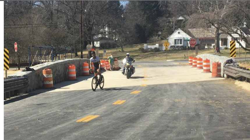
Construction along Beach Drive over Silver Creek finished ahead of schedule. The bridge reopened on 3/15/22.
