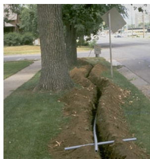
Trenching can kill trees causing them to become safety hazards along roads and sidewalks
