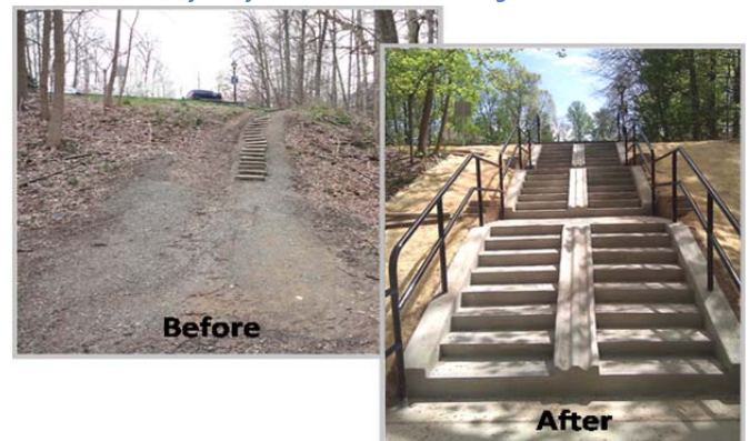
Rippling Brook Dr across Matthew Henson Trail 350 linear feet of new sidewalk with bike grooved stairs
