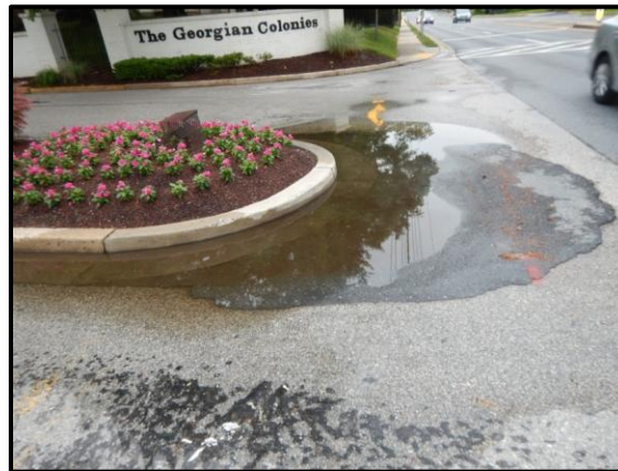
Water pools in the pedestrian crossing area.
