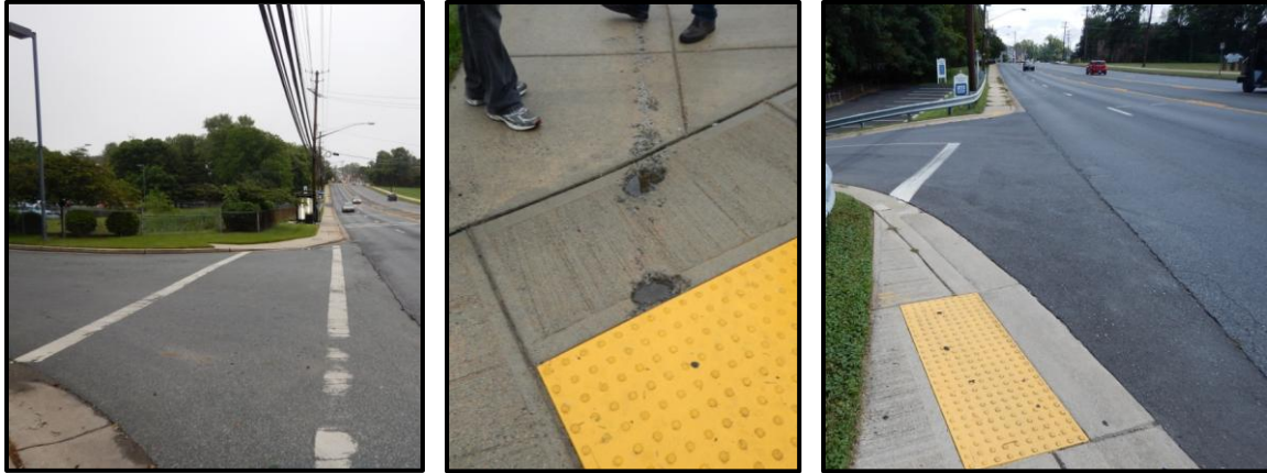
Left: Crosswalk is faded. Center: Damaged Sidewalk. Right: Pedestrian ramp is not aligned with pedestrian crossing path.
