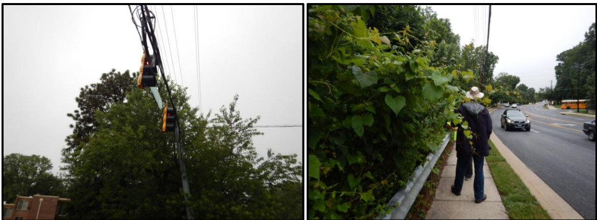
Left: Overhead utility lines block vehicular signal head at Homecrest Road. Right: Overgrown vegetation impedes the sidewalk.
