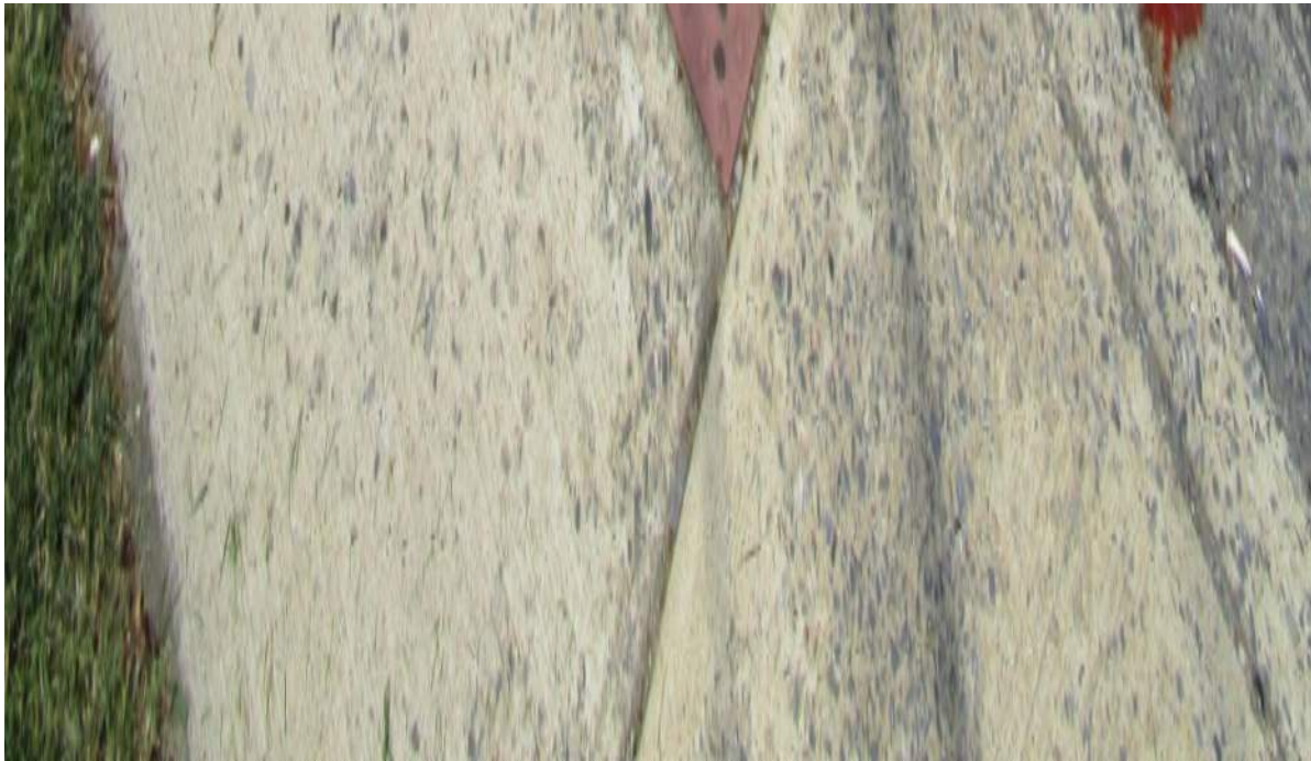
Photo 5.04. Curb and sidewalk damage – SW corner of Home Depot driveway.
