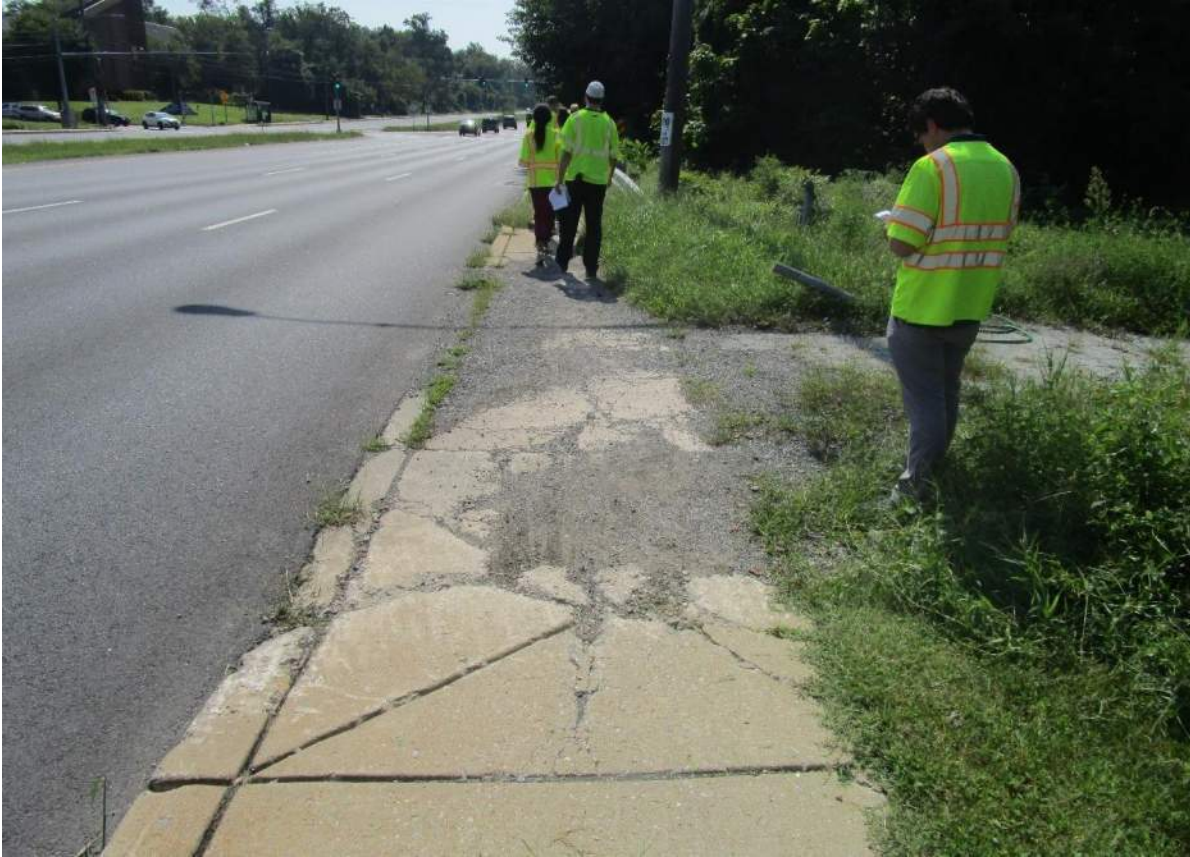
Photo 13.01. Damage and sediment at maintain access along SB MD 97, north of Hewitt Avenue.
