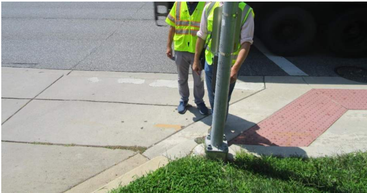
Photo 3.11. Pedestal pole less than 18" from curb face – NE corner of Postgate Terrace.
