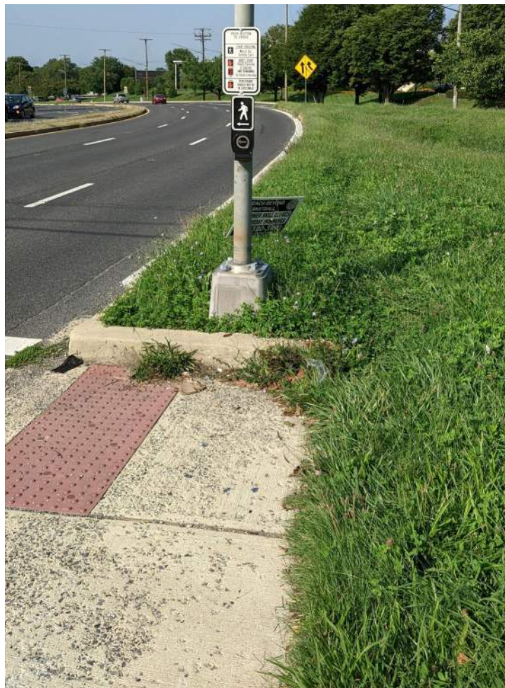
Photo 6.04. Grass sprawl onto sidewalk – NW corner of MD 97 at MD 185.
