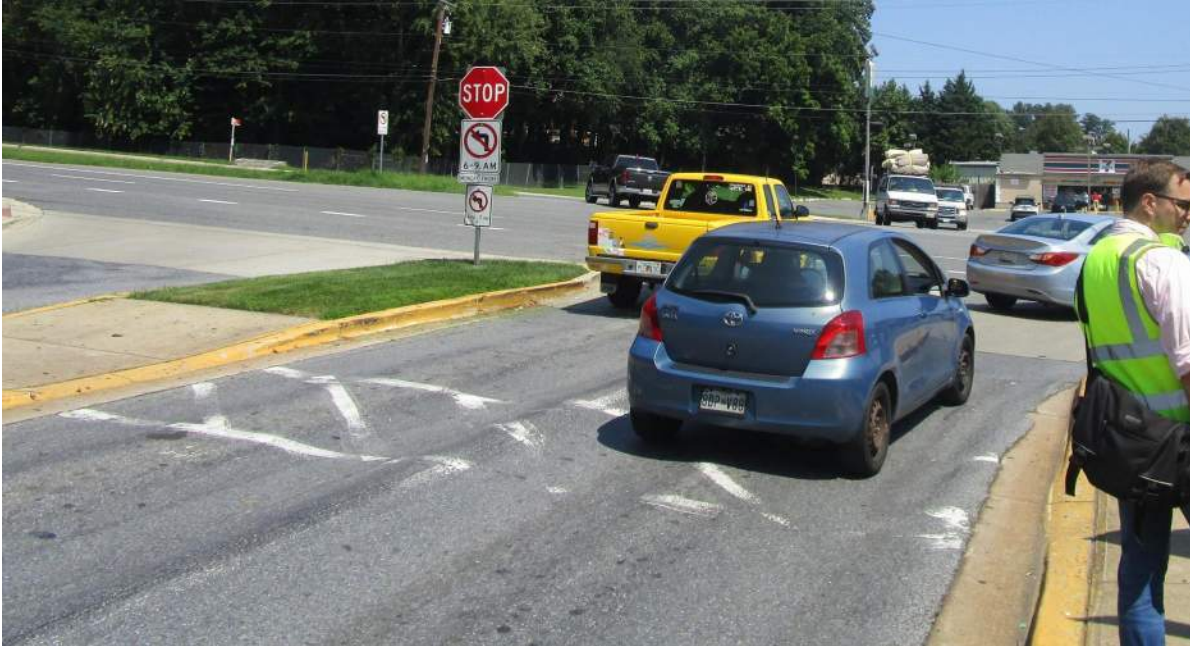
Photo 5.10. Home Depot driveway pavement condition.
