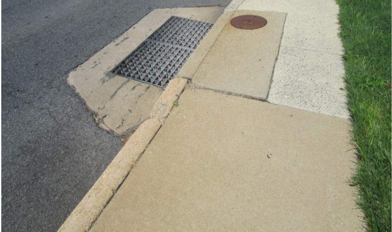
Photo 9.02. Damaged storm inlet / curbing along NB MD 97 near northernmost Aspen Manor driveway.
