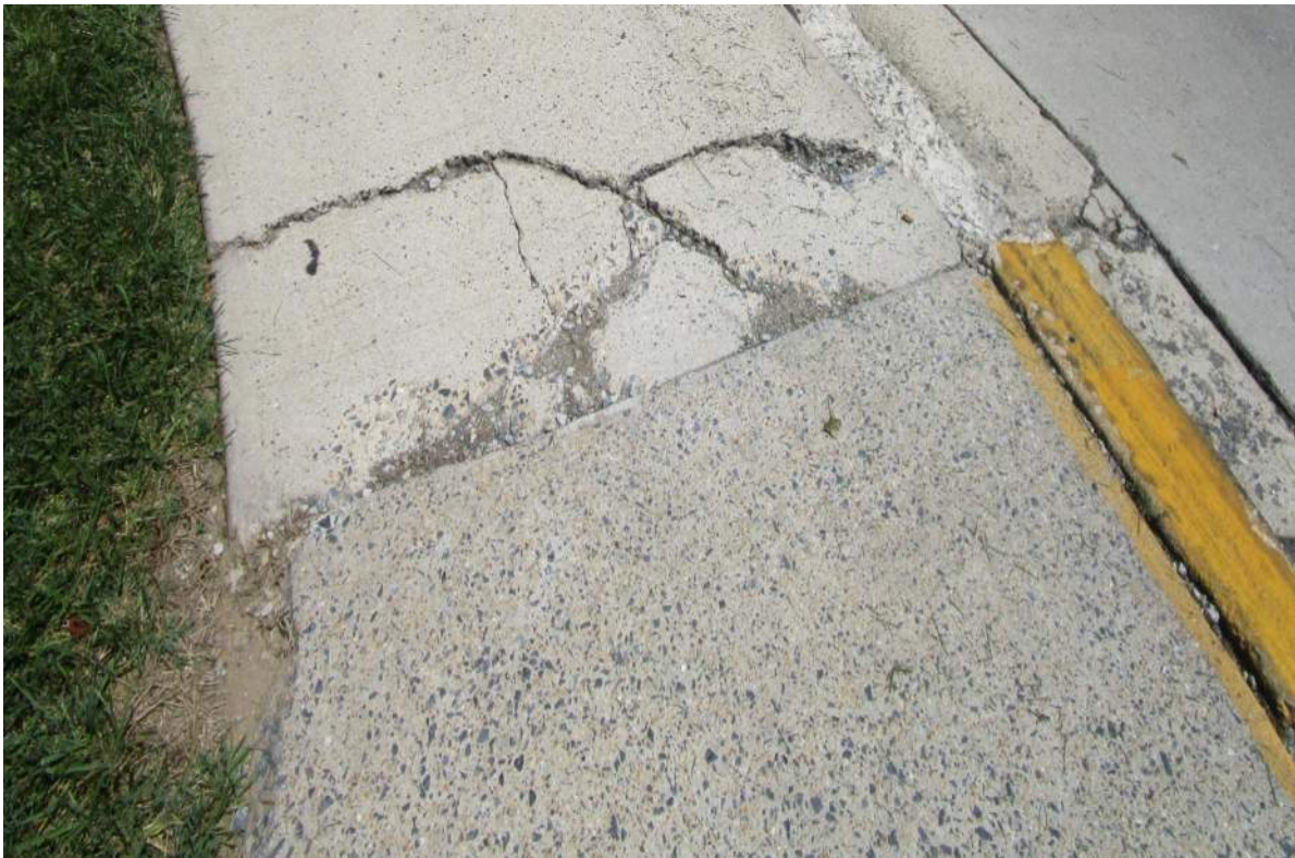
Photo 5.09. Sidewalk damage – NW corner of Home Depot driveway.
