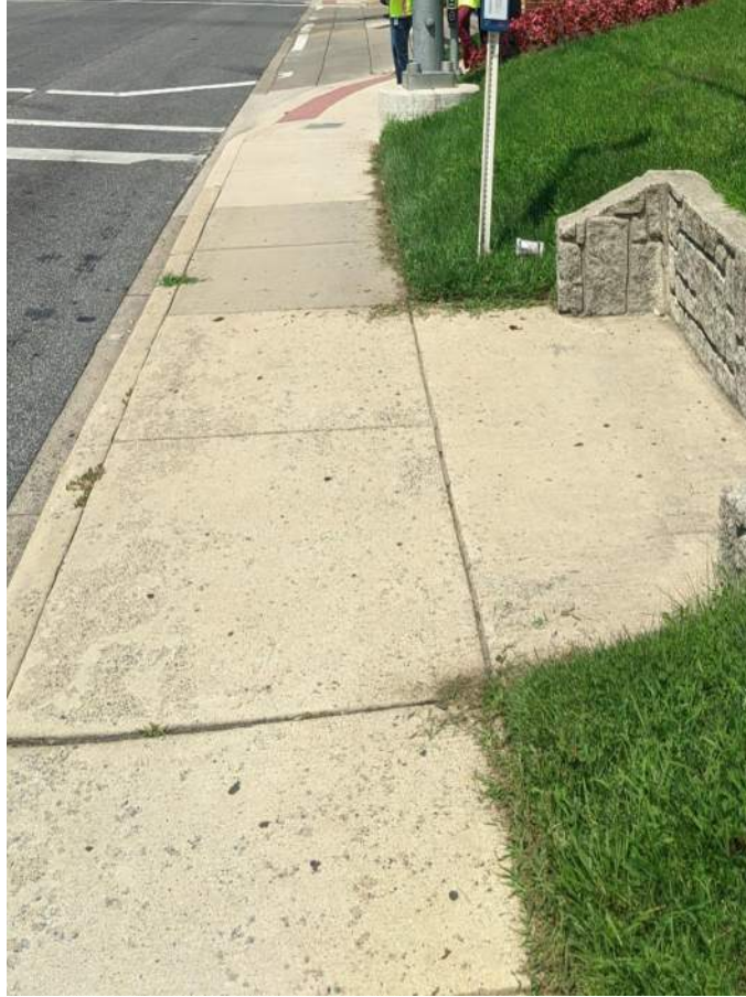
Photo 3.05. Sidewalk surface chipping – SE corner of Postgate Terrace.
