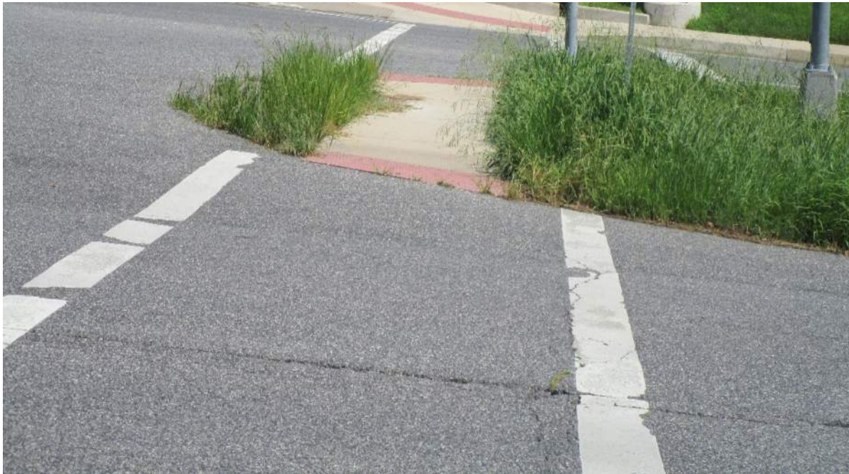
Photo 3.15. South median cut thru and nose – MD 97 at Heathfield Road / Postgate Terrace.
