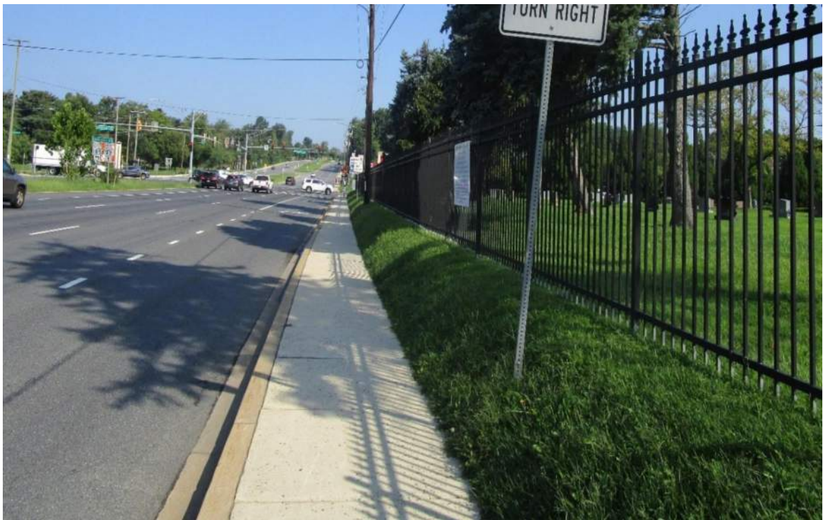
Photo 7.02. Sign support slipping and sign tilting.
