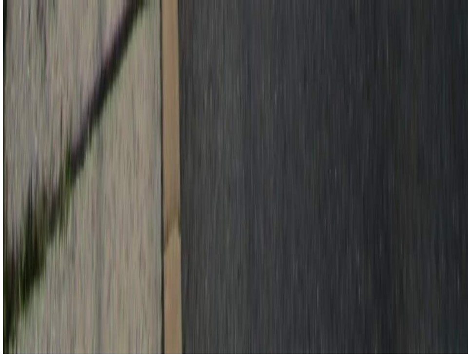
Photo 7.03. Vertical discontinuities in sidewalk along NB MD 97, near Aspen Hill Rd.
