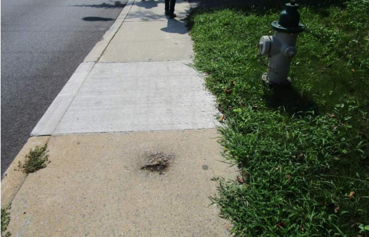
Photo 11.01. Sidewalk damage – SB MD 97 near Ralph Road.
