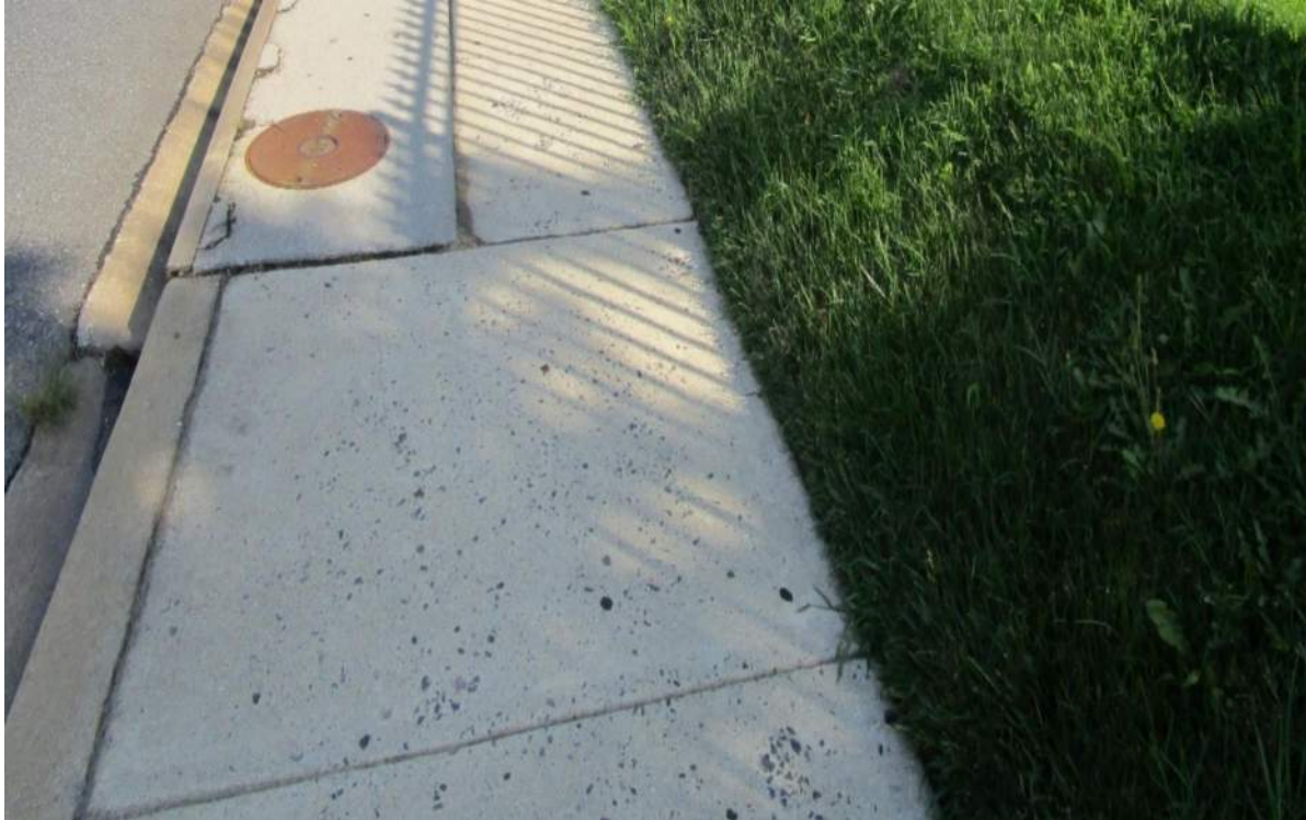
Photo 7.05. Storm inlet structure is not flush with sidewalk – NB MD 97 near MD 185.
