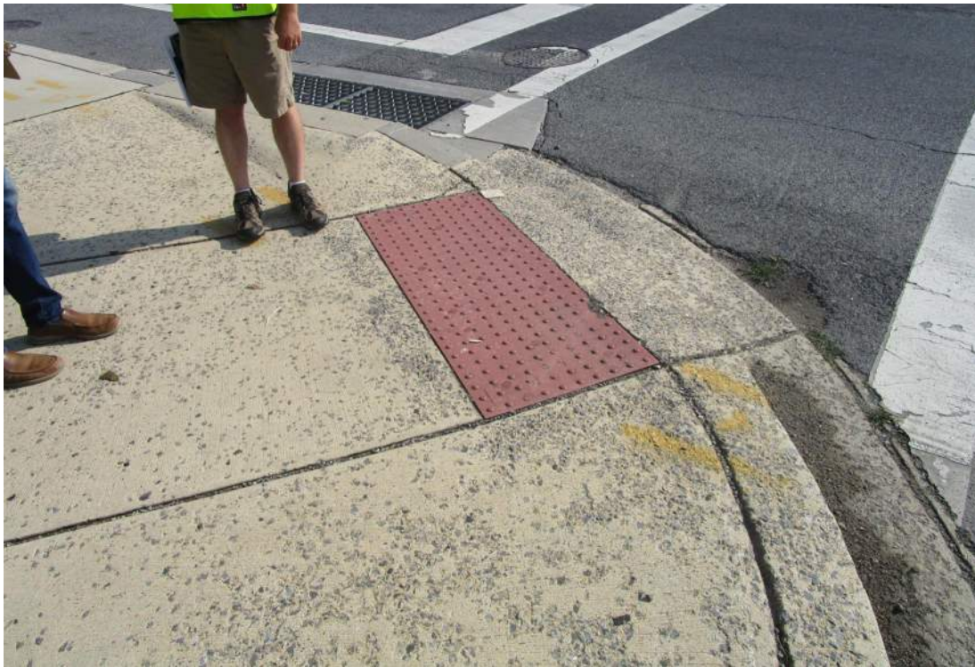
Photo 6.06. Sidewalk in poor condition – NW corner of MD 97 at MD 185.
