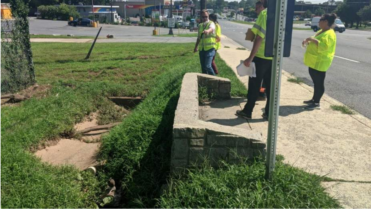
Photo. 5.05. Critical slope behind bus stop (WMATA ID 2000892).
