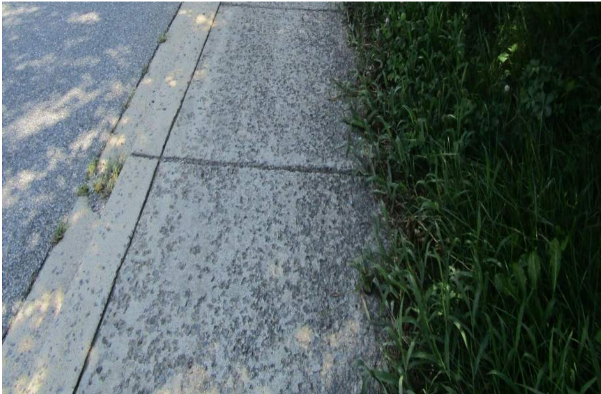
Photo 3.03. Sidewalk surface chipping along SB MD 97.
