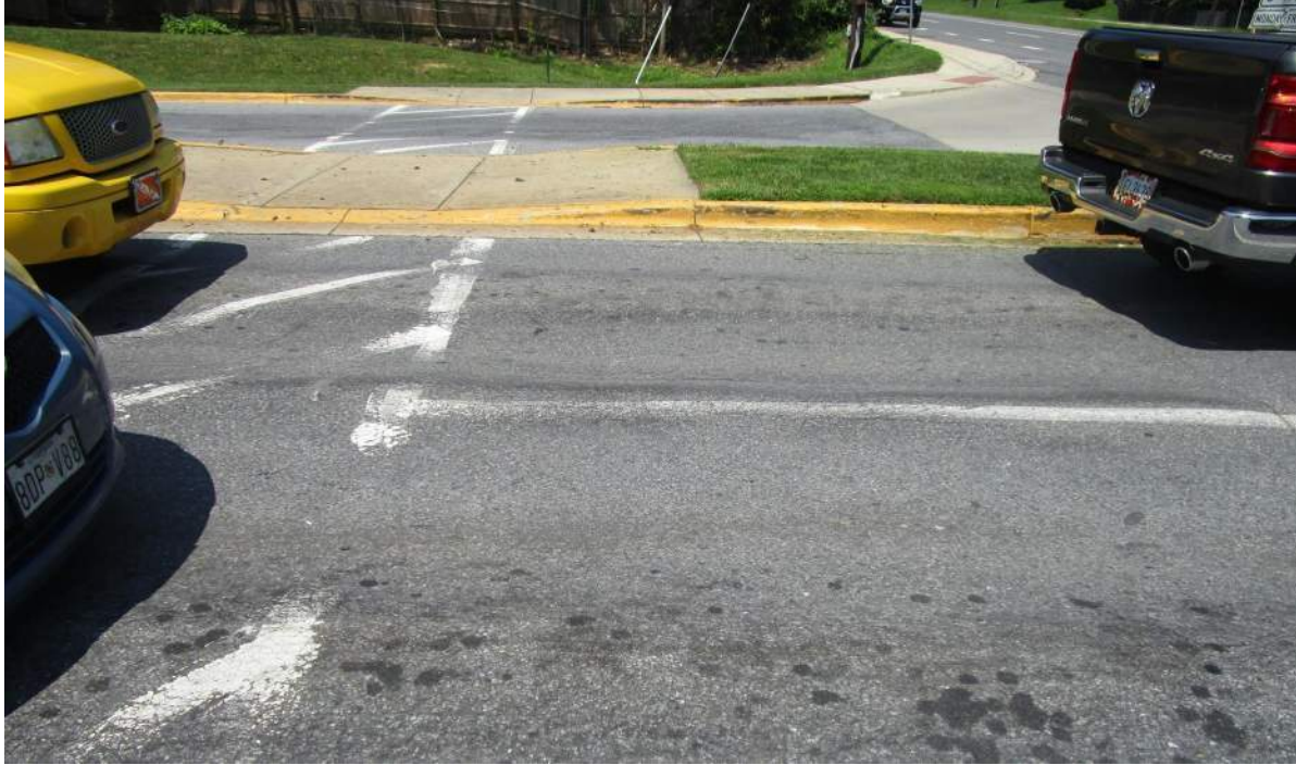
Photo 5.03. Non-compliant crossing offset from driveway apron – Home Depot.
