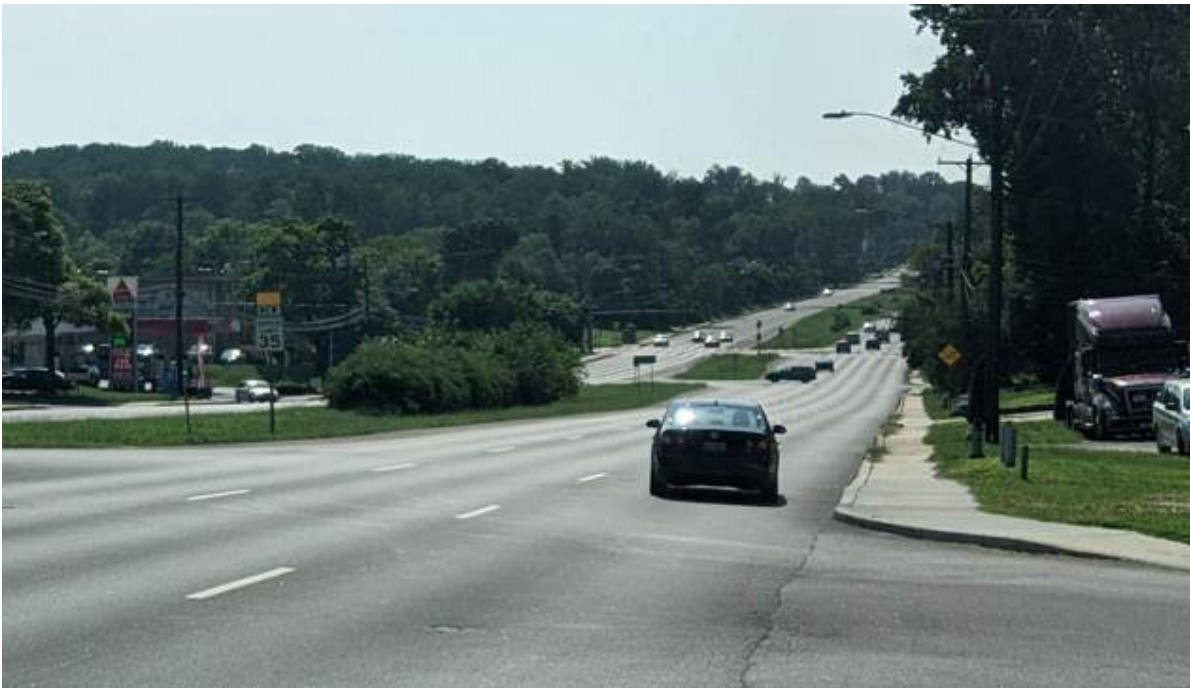
Photo 11.02. Missing speed limit sign on right.
