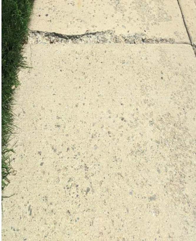
Photo 2.07. Damaged sidewalk along MD 97 NB.
