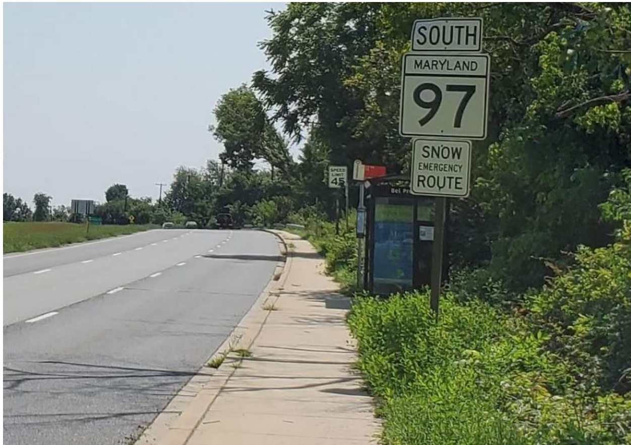
Photo 2.06. WMATA ID 2000913. Bus shelter with broken audio message button.
