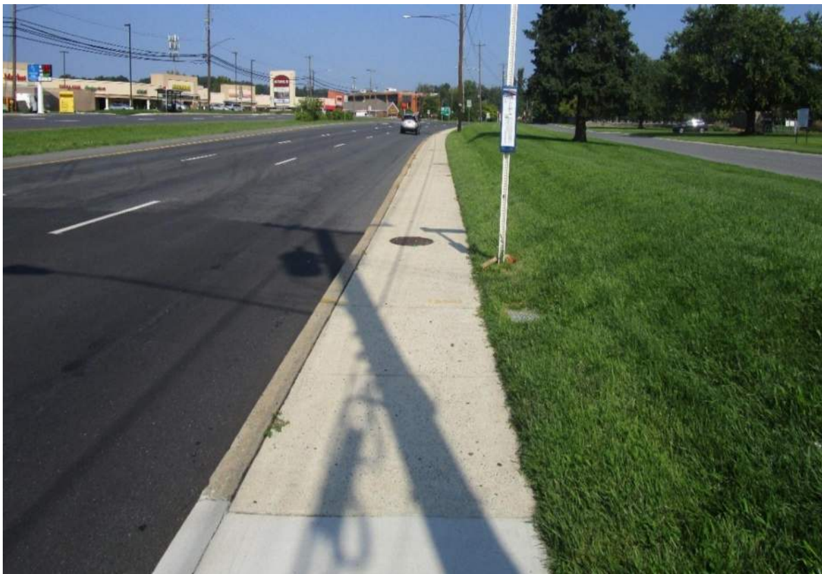
Photo 7.06. Missing ADA bus pad at bus stop (WMATA ID 2000864).
