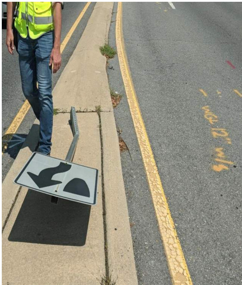
Photo 1.06. Damaged sign – east median of Bel Pre Road.
