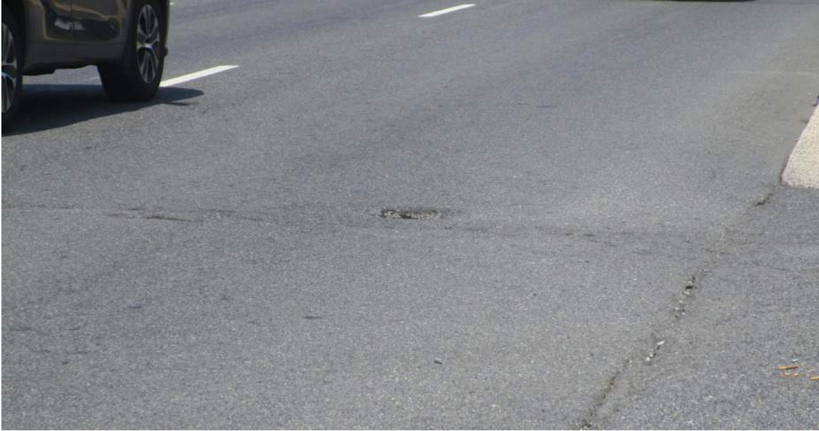
Photo 9.04. Pothole in roadway – NB MD 97.
