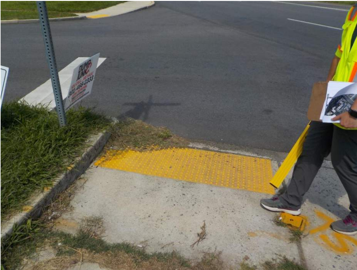
Photo 10.01, 10.02. Unmarked crossing of Wendy Lane. Sediment and growth in sidewalk.
