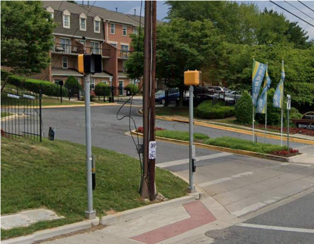
Photo 3.02. Wiring hanging off PEPCO pole #
