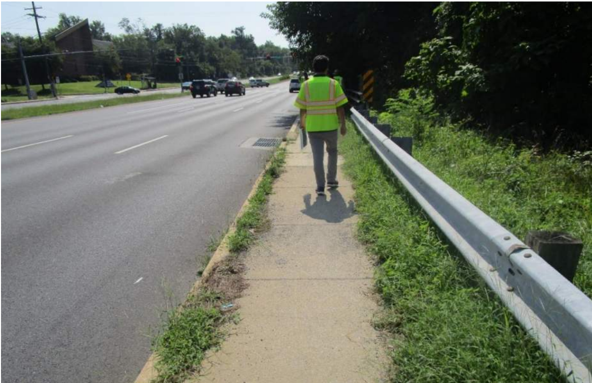
Photo 13.02. Grass sprawl and growing out of sidewalk joints – SB MD 97.
