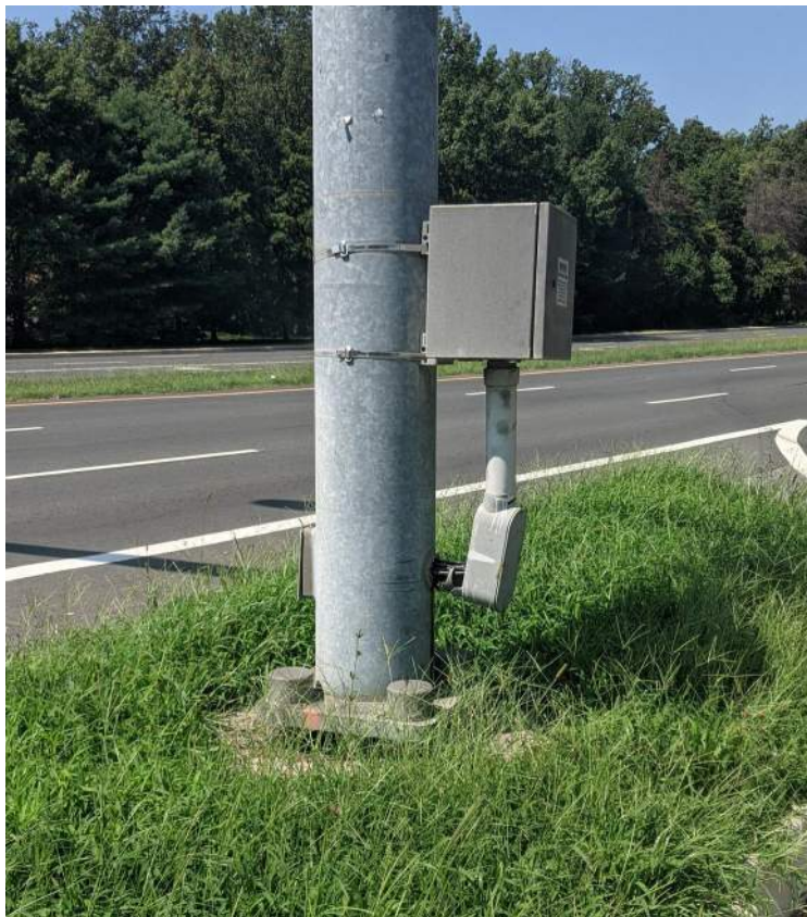
Photo 1.08. Broken conduit – NE corner of Bel Pre Road.
