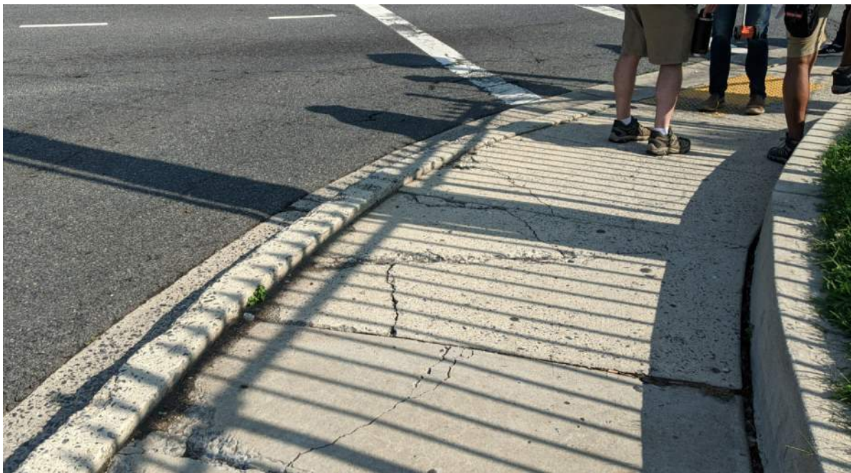
Photo 6.13. Damaged sidewalk and curb – SE corner of MD 97 at MD 185.
