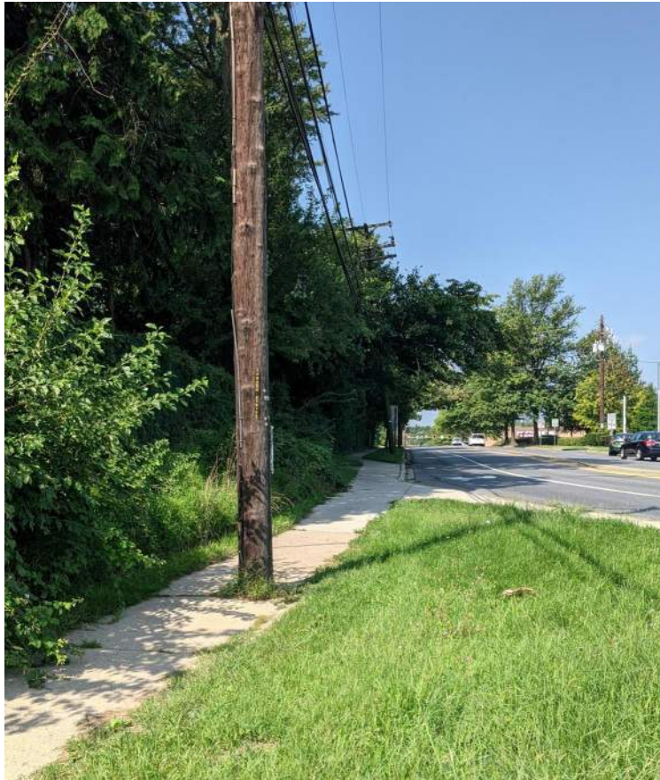
Photo 8.10. Utility pole creating ADA pinch point in sidewalk – SW corner of Aspen Hill Road.
