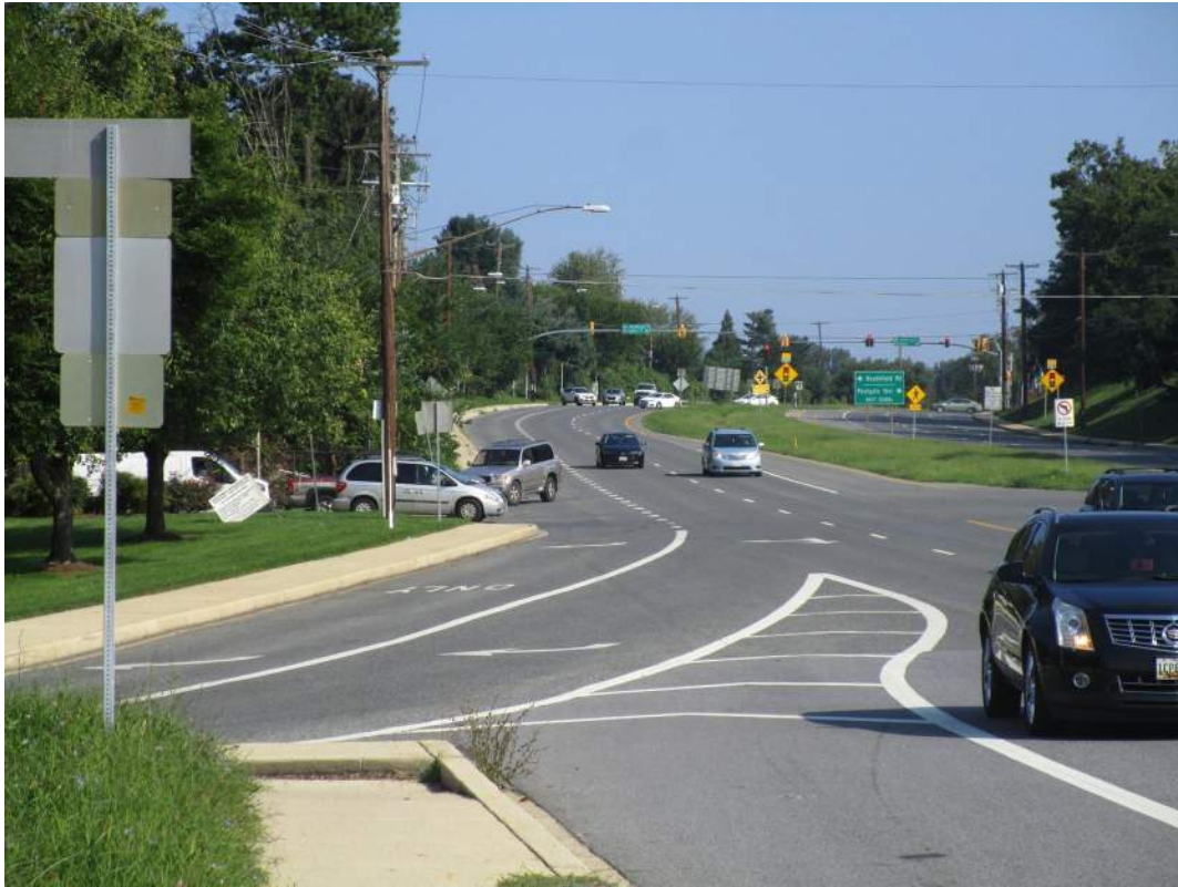
Photo 6.05. Channelization nose missing object marker.
