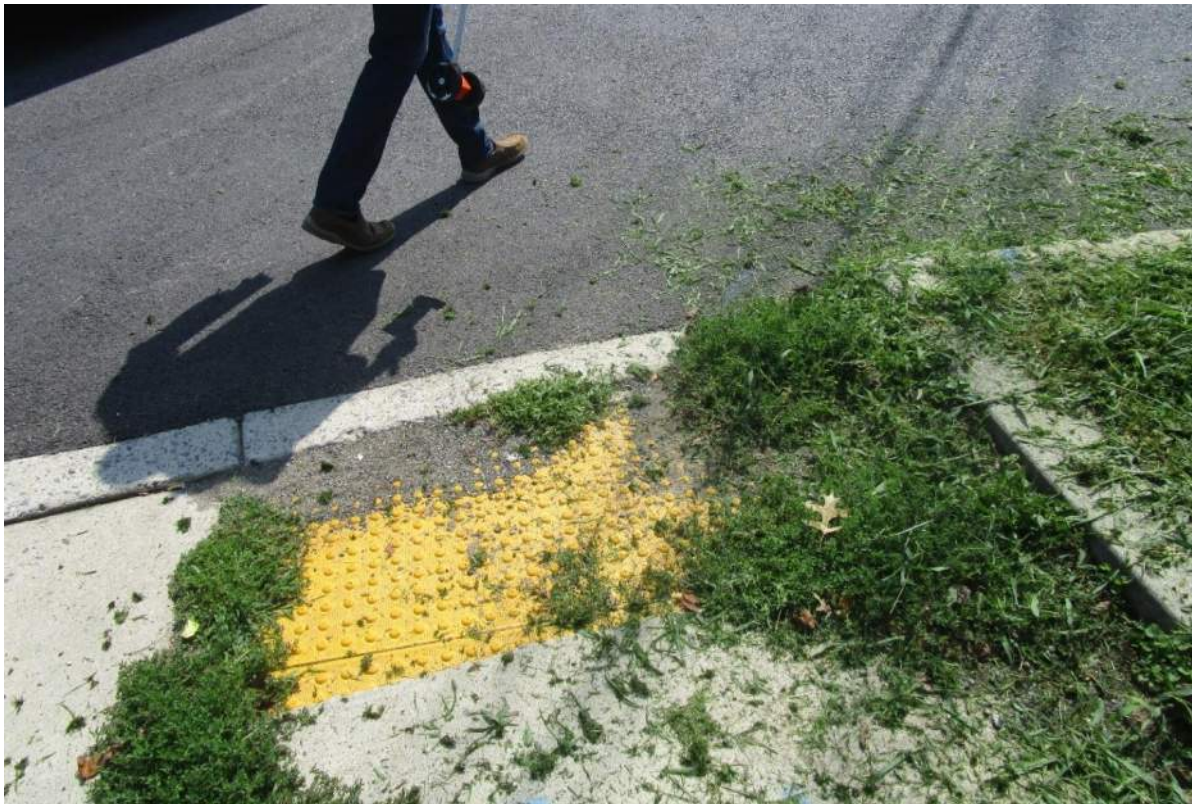
Photo 12.02. Grass growing in sidewalk joints – SW corner of Ralph Road.
