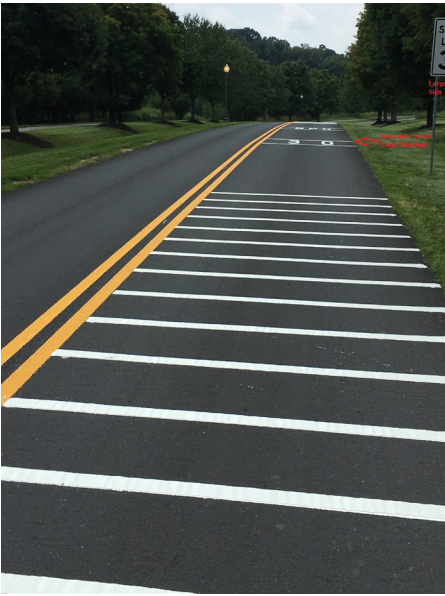
Figure 8-11. Example of optical speed bars
