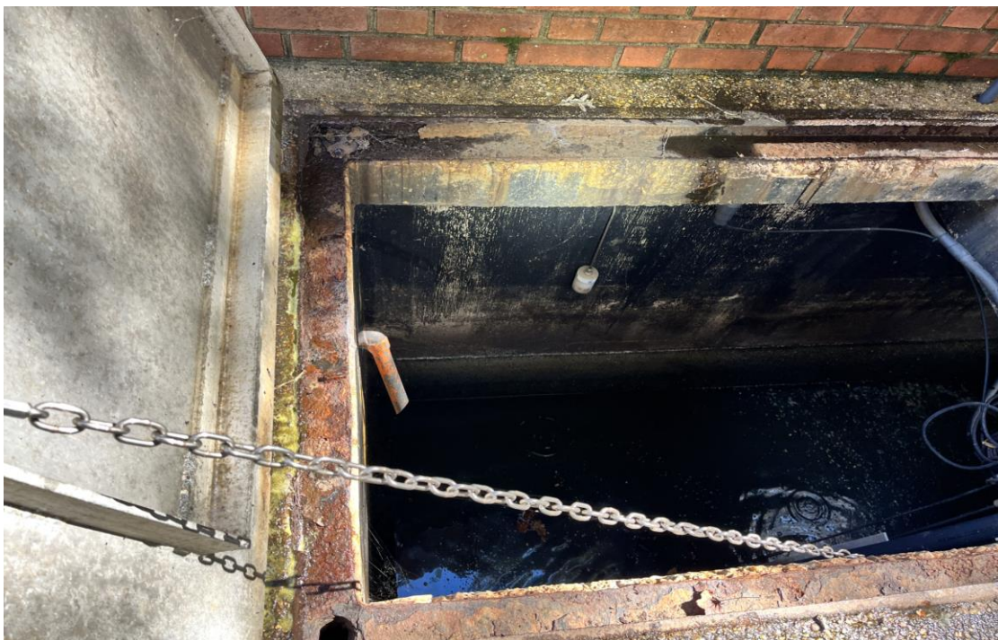
Arcola WWPS wet well and the conduit for possible tube insert.
