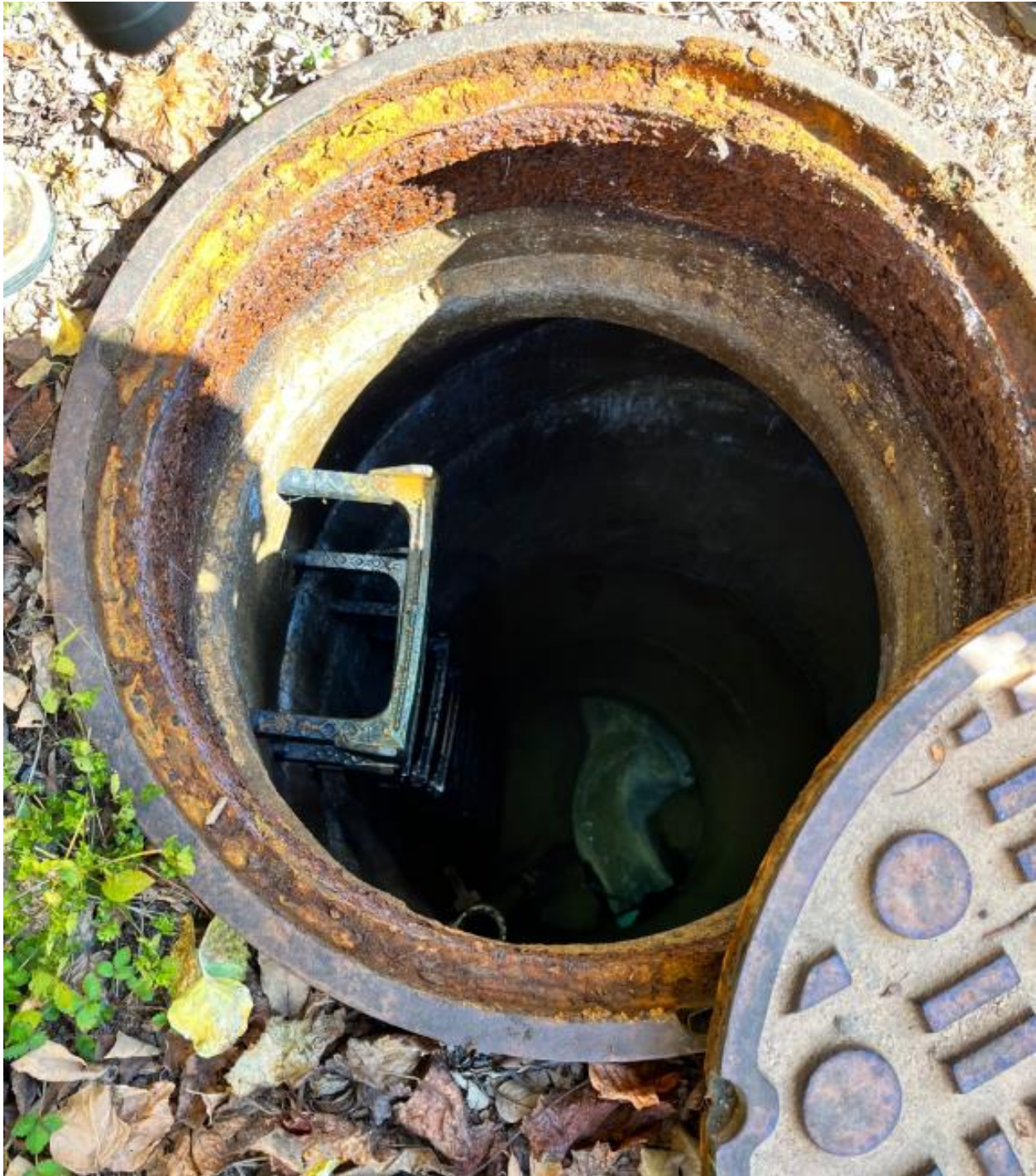
From Top – View into the manhole adjacent to King farm WWPS. Sewer running into the pump station.
