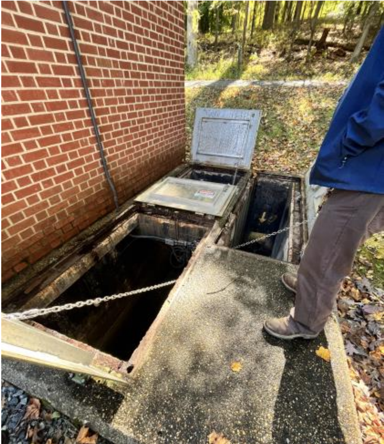
Arcola WWPS wet well top view.
