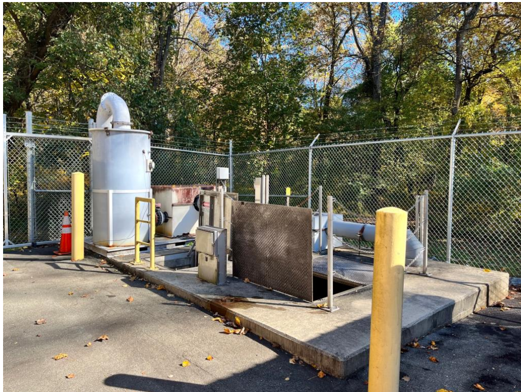
North Branch WWPS wet well entrance
