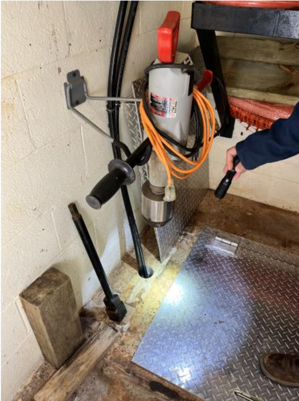
The ground level floor for composite unit placement and the conduit for tubing.
