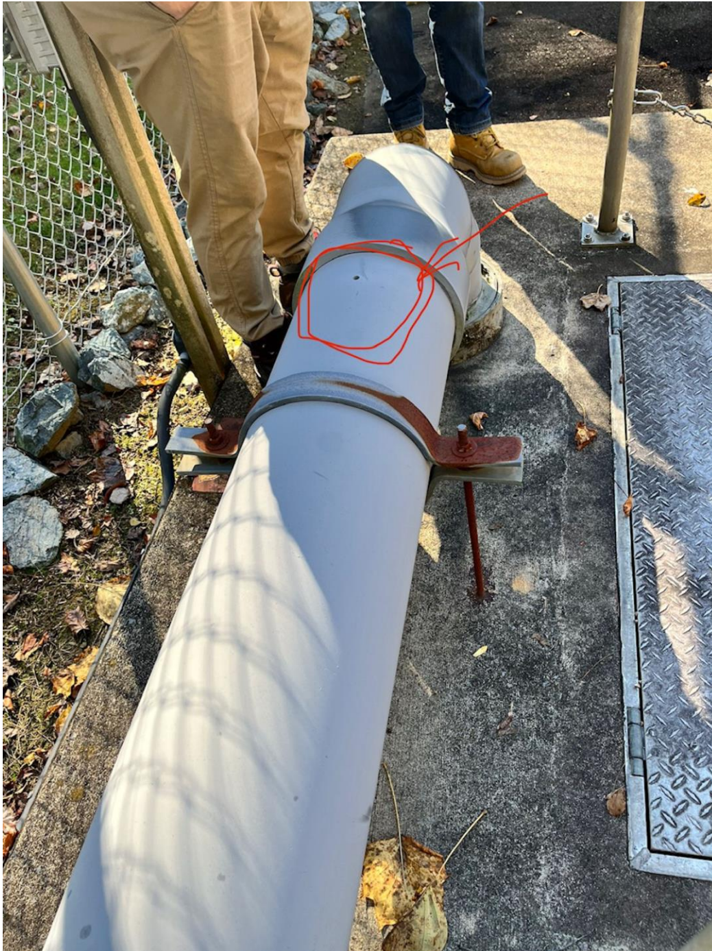
North Branch wet well air supply pipe as the possible access point for sample tube line.
