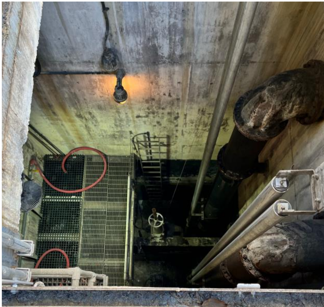
From Top - View into the well at King Farm WWPS
