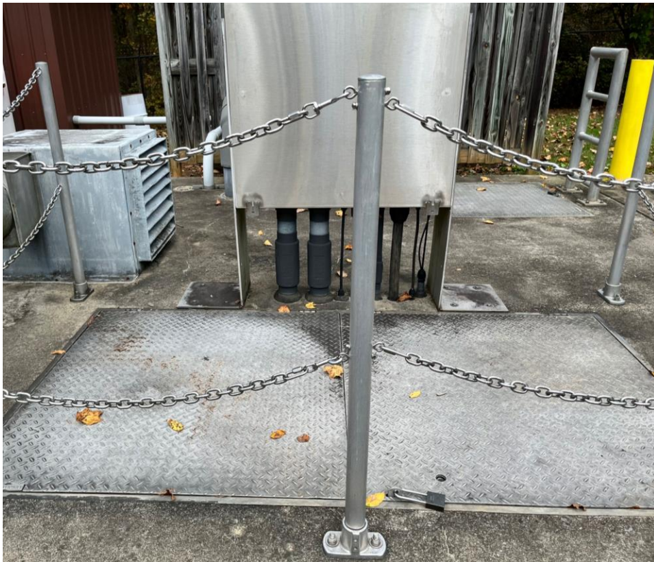
Hoyles Mill wet well access point.
