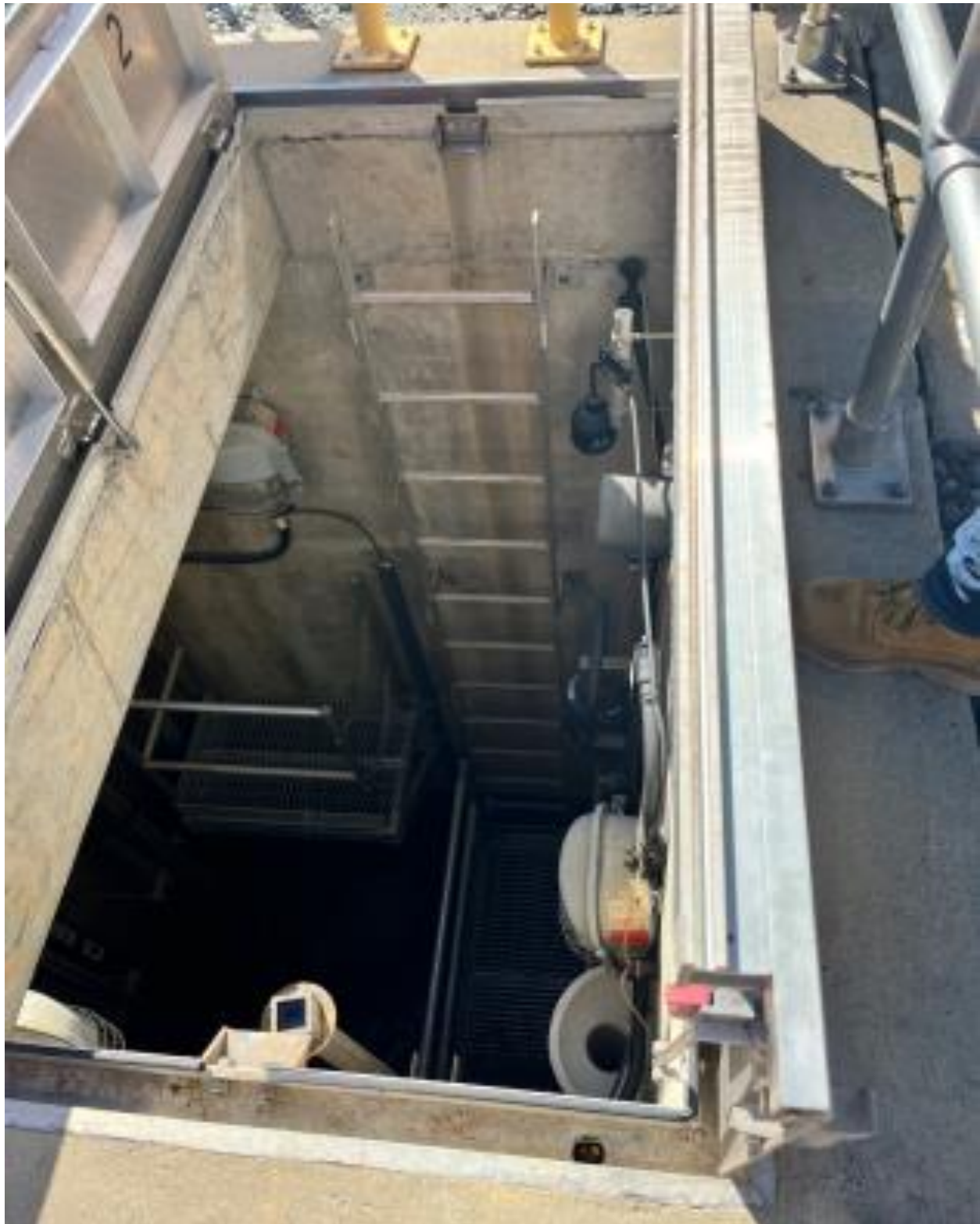
North Branch WWPS wet well entrance
