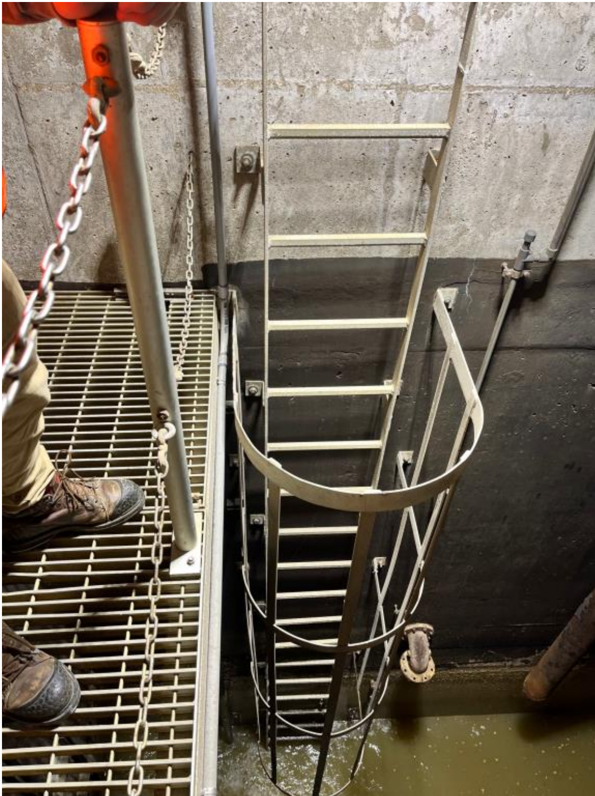
Deep wet well at Hoyles WWPS
