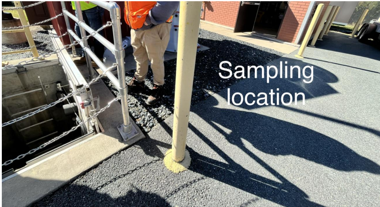
Deep wet well access at Rock creek wastewater pump station (WWPS)
