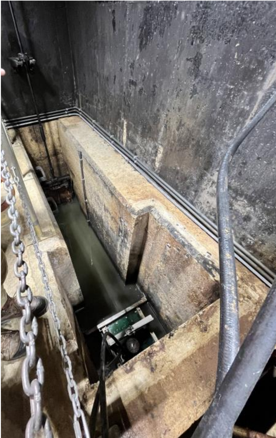
Wet well at Reddy Branch WWPS
