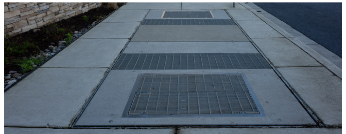
Figure 3-13. Example of grates that may present tripping hazards
