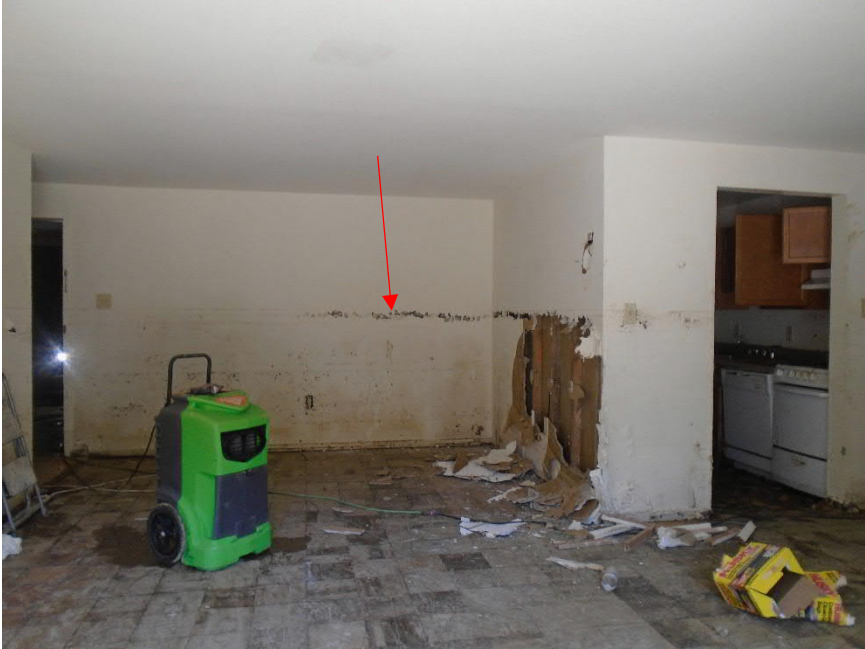
Figure 35 - High Water Mark Building 8
