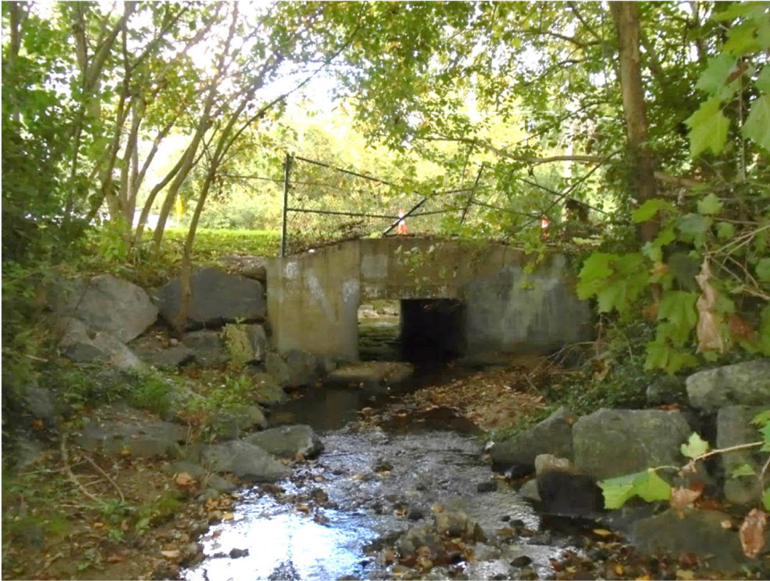
Figure 53 - Atlantic Avenue Crossing Tributary 2. Note: Damaged fence from flooding.
