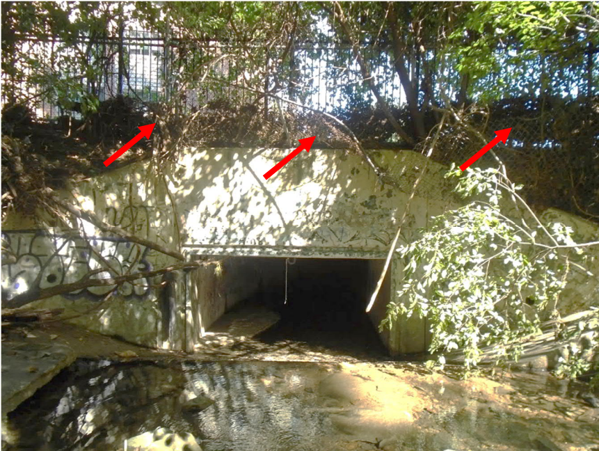
Figure 57 - Tributary 2 Culvert Headwall. Note Debris in Fence (Arrows).
