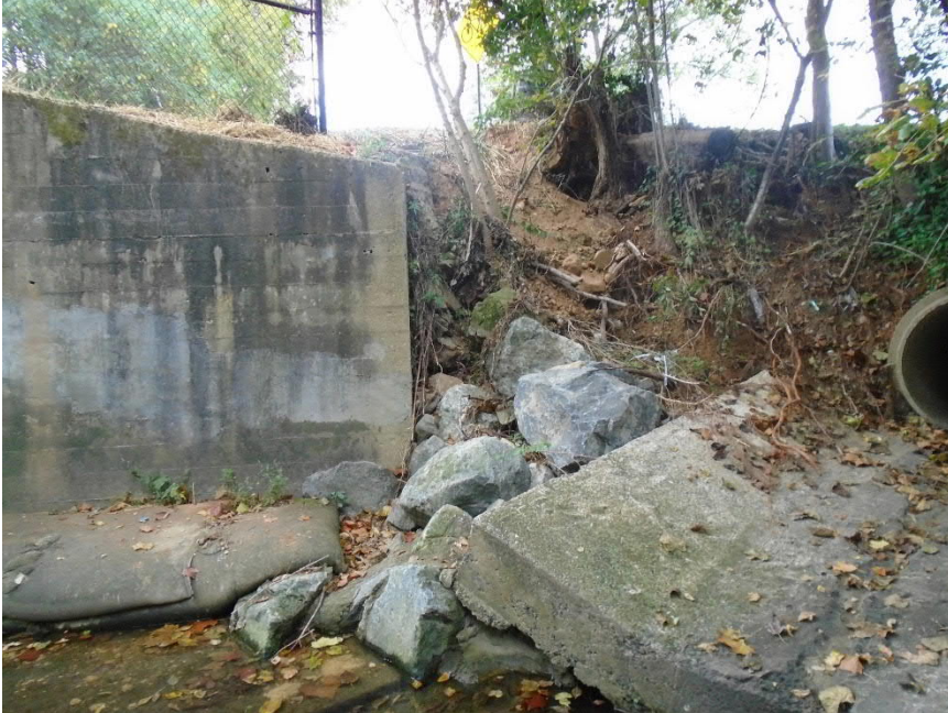
Figure 54 - Debris and Erosion at Atlantic Avenue Crossing.
