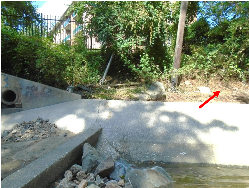
Figure 62 - Typical Erosion Along Bank Above Concrete Apron.
