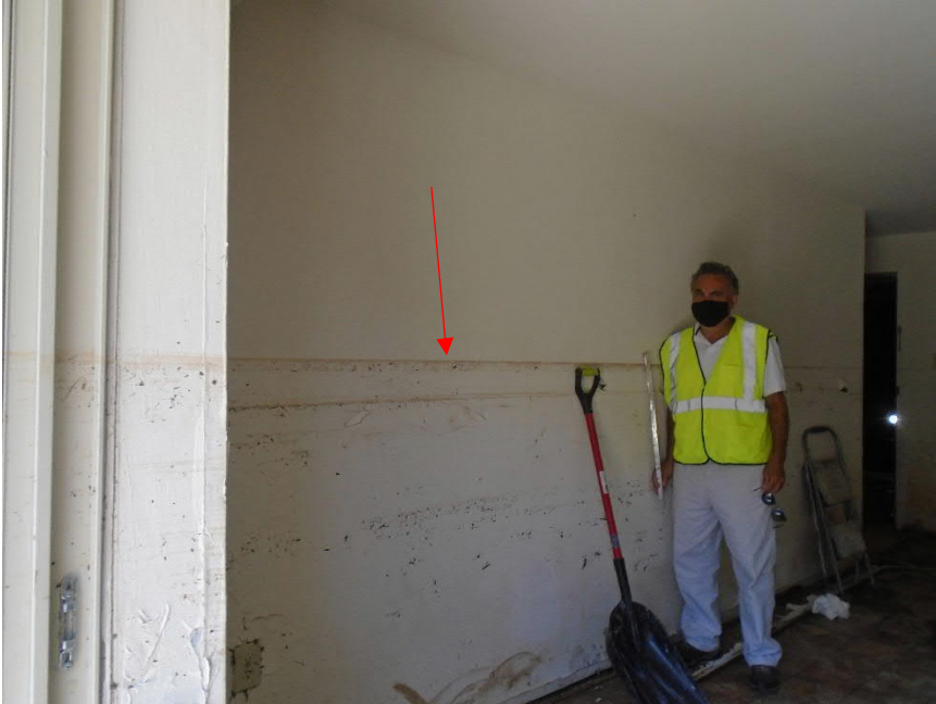
Figure 36 - High Water Mark Building 8
