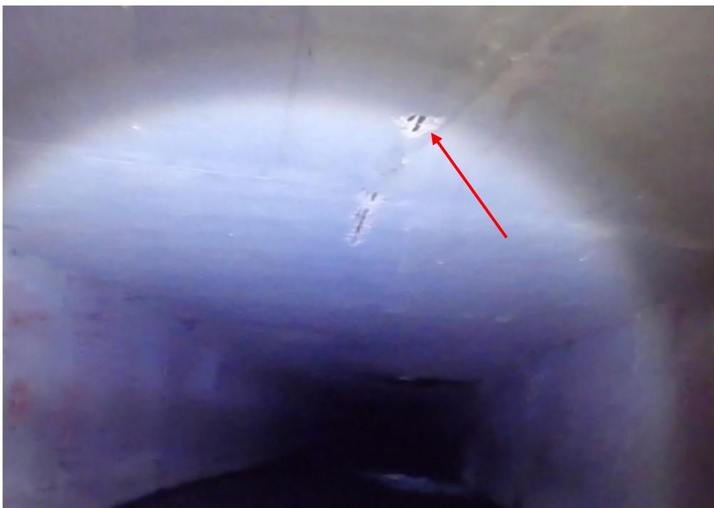
Figure 23 - Typical Minor Spall with Exposed Reinforcing Steel on Top Slab of Box Culvert
