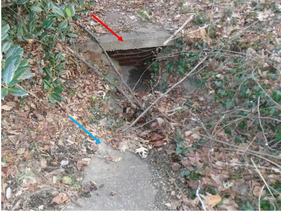
Figure 70 - Downstream end of concrete flume (blue arrow) connected to inlet (red arrow) at the west end of the apartment complex.
