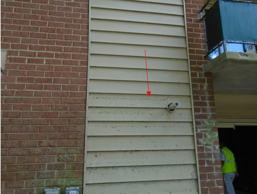
Figure 37 - High Water Mark Building 7
