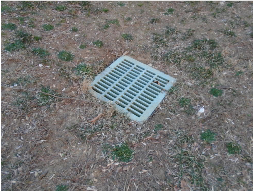
Figure 40 - Inlet with Plastic Grate in Depression of Rock Creek Woods Apartments
