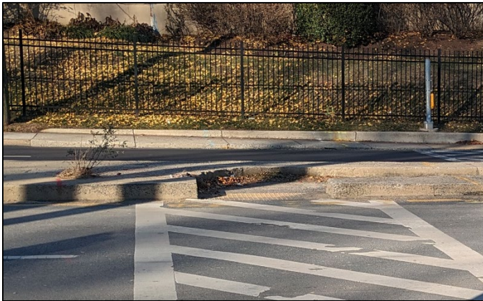
Figure 16. HIB Equipment Damage
