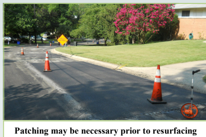
Patching may be necessary prior to resurfacing
