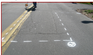
Typical paint markings
