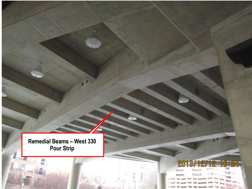
Image 10: Additional Beams for Remediation of Shear and Torsion Deficiencies per KCE and IAC Recommendations
