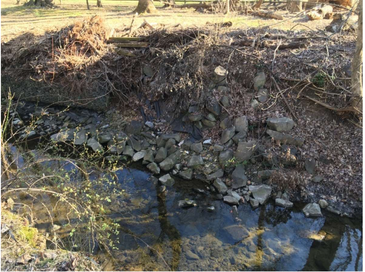
(Above: along an adjacent private property, a failed attempt at stream bank stabilization with Gabion baskets and rip rap along Old Farm Creek Tributary, North Bethesda)
