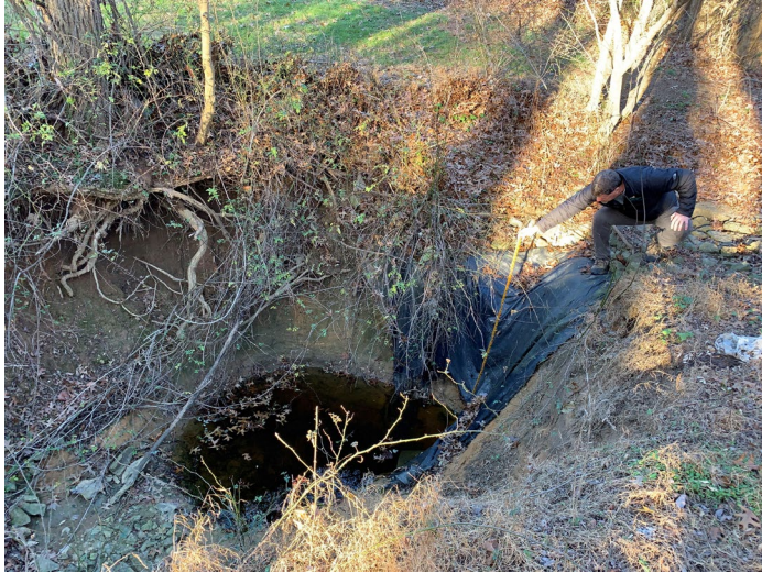
Photo 2: Upstream limits of Erosion Channel
