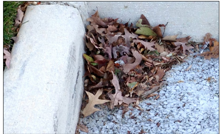
White Oak Community Center pervious concrete parking lot. Typical maintenance: Remove leaf debris.
