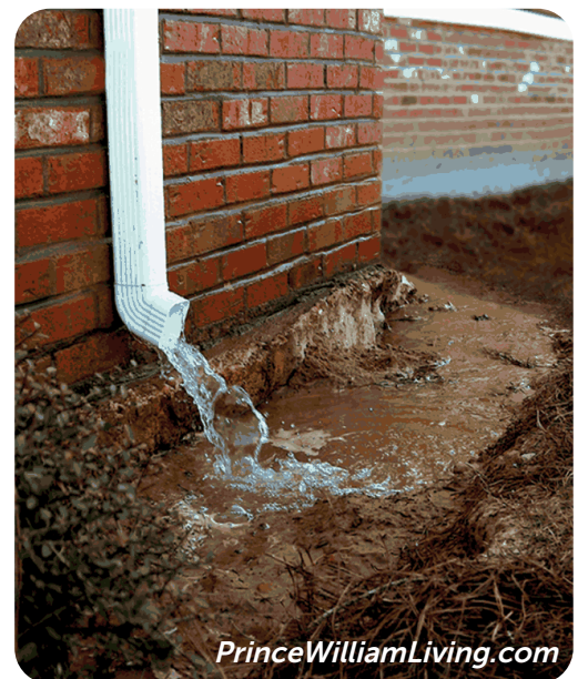
An example of downspout-related erosion and stormwater problems. This could be solved with a Stormwater Garden.
