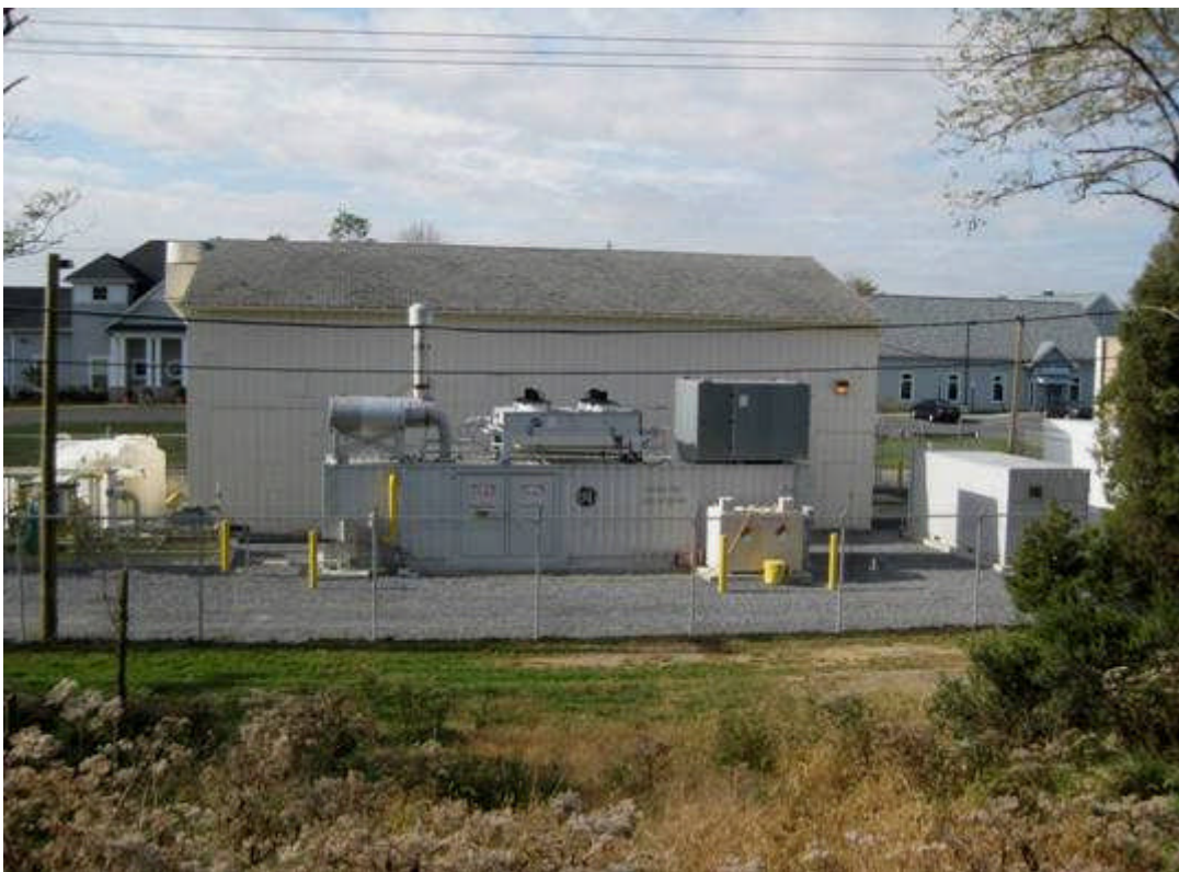
Photo 4 – Landfill Gas-to-Energy Facility
