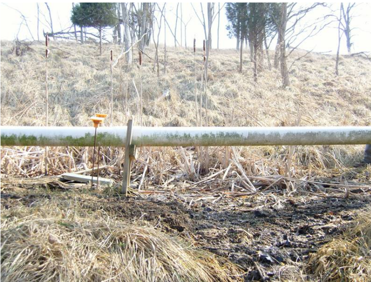
Photo 6 - Leachate Seep (before repairs)
