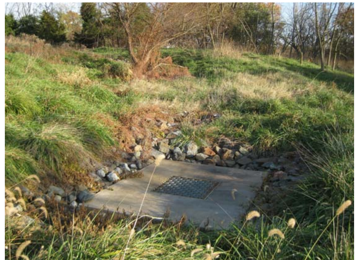
Photo 5 – Concrete Inlet with upslope Drainage Channel for Stormwater Collection
