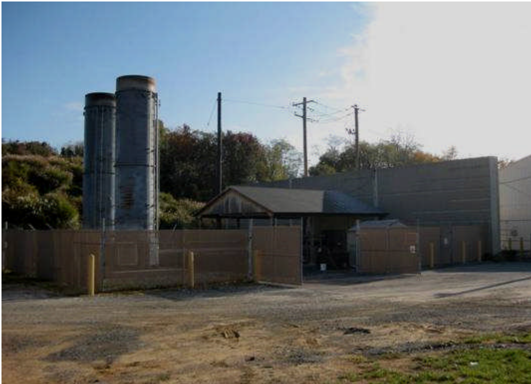
Photo 3 – Landfill Gas Flare Station
