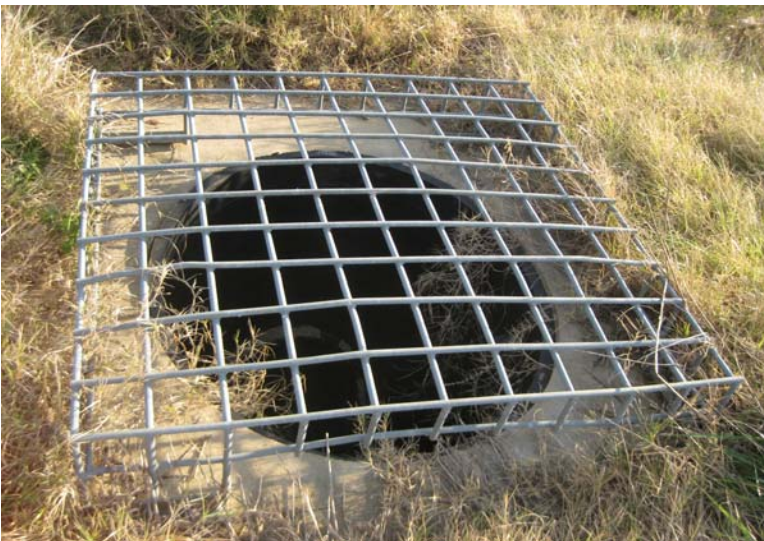
Photo 4 – HDPE Manhole with upslope Drainage Channel for Stormwater Collection
