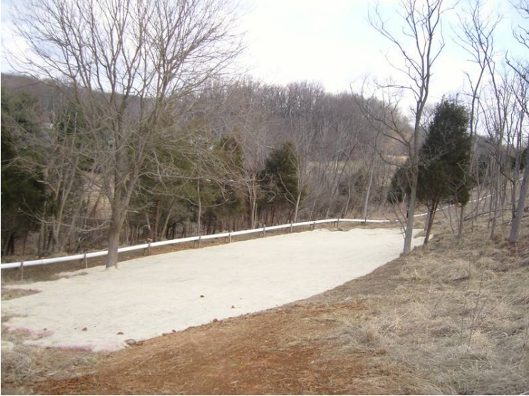
Photo 8 – Disturbed Area of Leachate Seep (during repairs)
