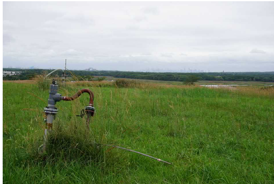
Methane Capture Station
