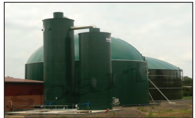
Example of an anaerobic digester that processes food scraps and other organic materials deemed acceptable by the operator.
