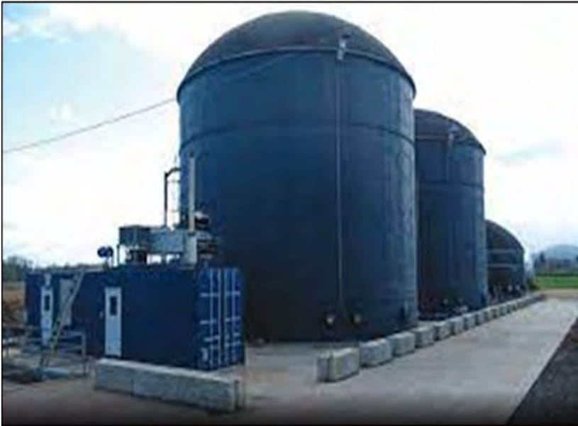
Anaerobic Digestion with RNG from Biogas
