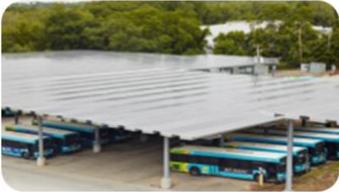
1. 5.5 MW Solar PV Canopy
