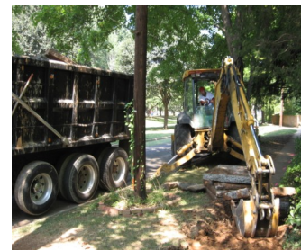
Defective concrete is removed
