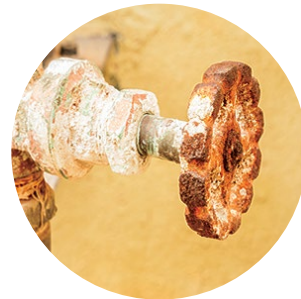
CHLORIDE corrosion, salty taste
