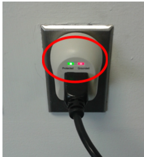
Figure 5 - Picture of Red and Green Lights on the Surge Protector
