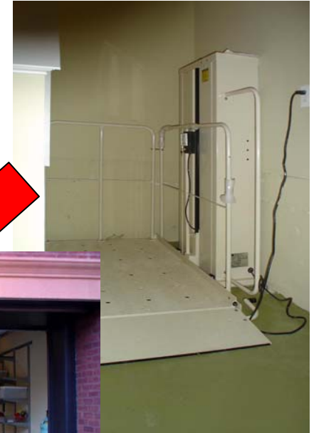
Stairlift in the garage
