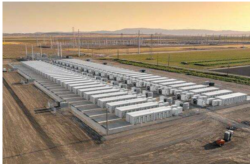
Exhibit 10, pg. 2 “Exhibit 5” – BESS Installations
