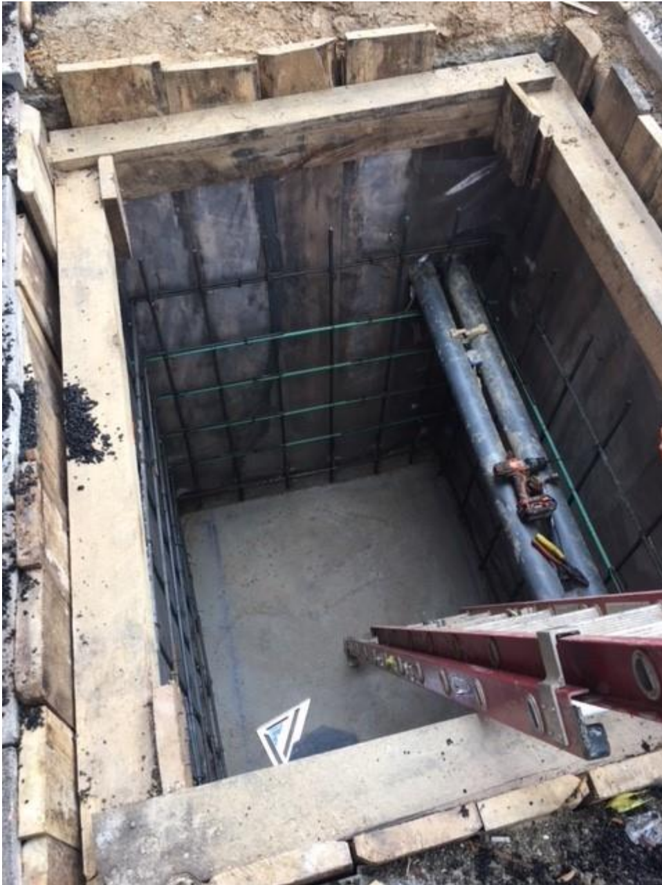
Work to be completed on the week of Aug 27, thus eliminating the need for daytime closures
