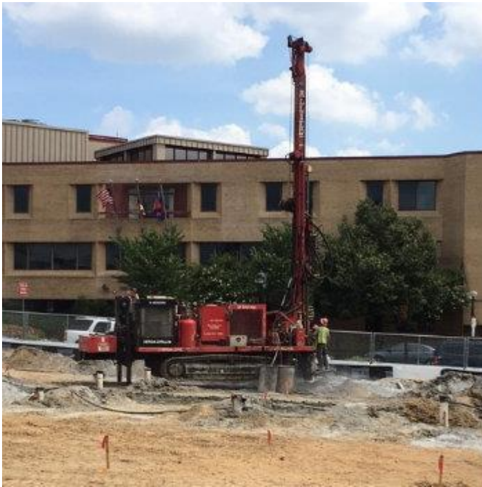
Typical Geothermal Drill Rig
