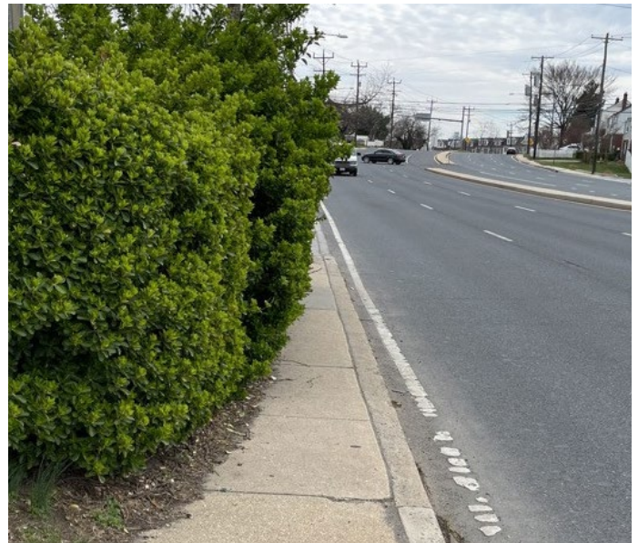
Figure 18: Example of vegetation overhanging sidewalk
