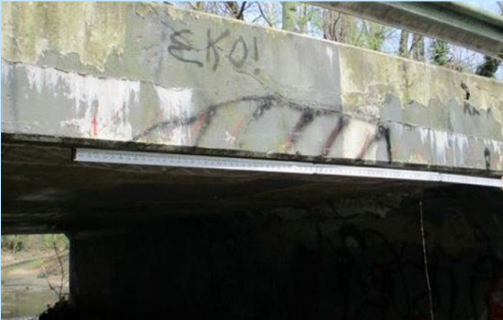
Delamination, Cracking, & Efflorescence at the South headwall & Top Slab of Cell No. 1
