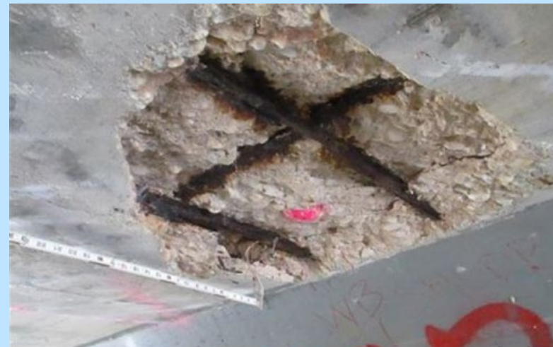
Exposed Reinforcement Cell 1 Top
