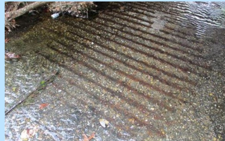
Exposed Reinforcement Cell 1 Bottom
