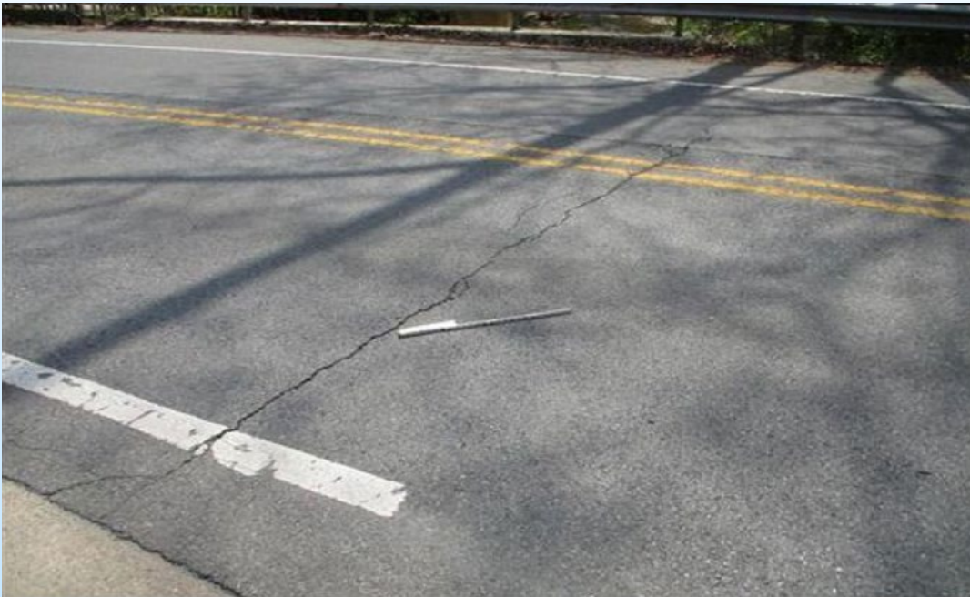
Crack in the Asphalt Pavement at Edge of Culvert (western approach)
