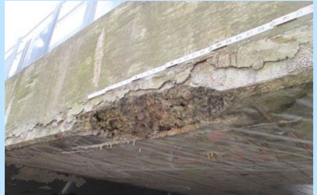
Spalling & Delamination at the North Headwall & Top Slab of Cell No. 1
