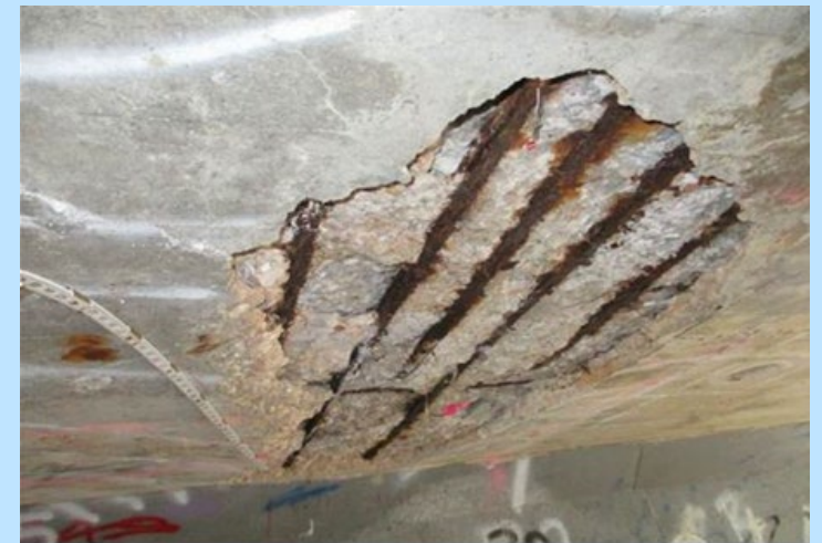
Exposed Reinforcement Cell 2 Top
