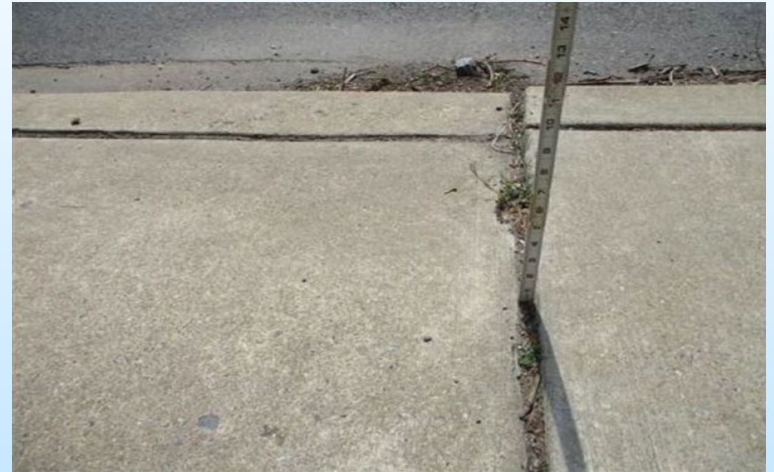
Northeast Approach Sidewalk Settlement Below Sidewalk Over the Structure
