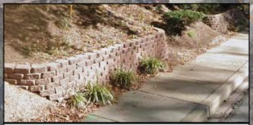
Inset 1 - Example of Segmental Block Retaining Wall (Jones Bridge Road in Bethesda)
