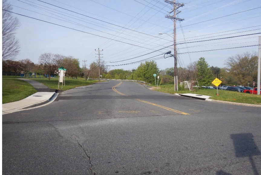
Photo 11 – Missing Stop Bar on South Approach
