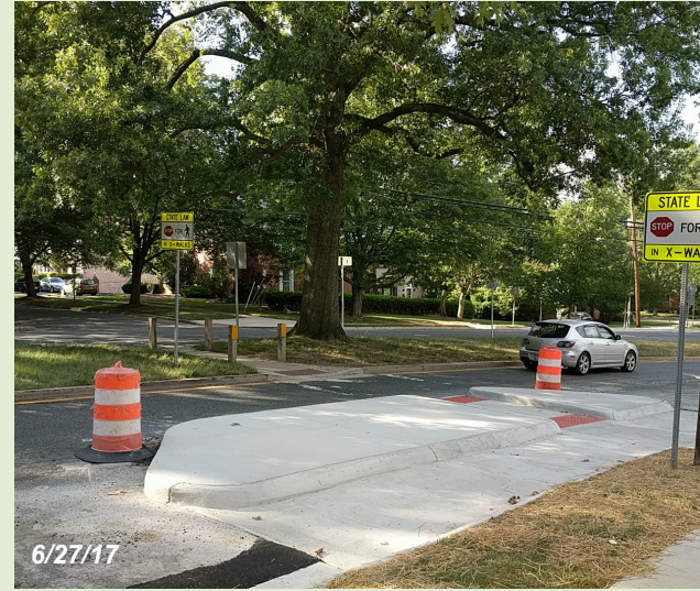
This island shortens the crossing distance and slows drivers along Spring Street at Woodland Way.
