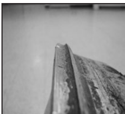
Photo 8. Severe rim flange wear.
