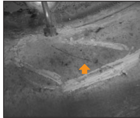
Valve hole crack
