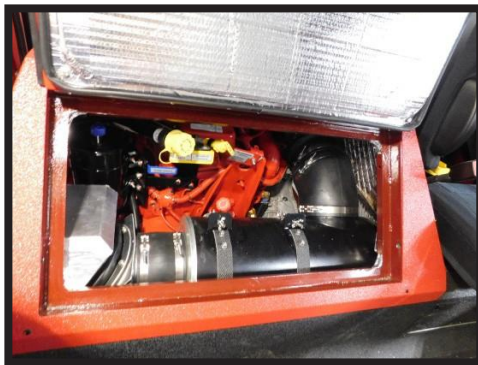
Access Door in rear of cab
