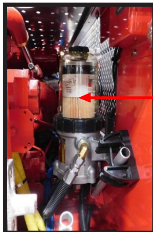
Primary Fuel Filter Filter/Water Separator
