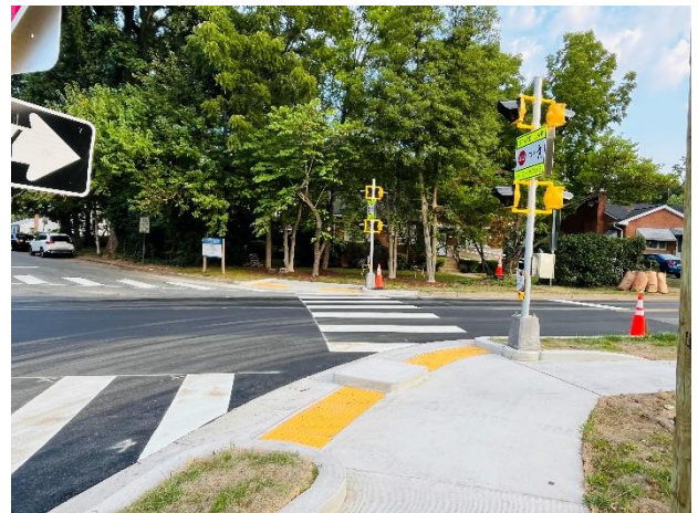
Figure 19 - New pedestrian beacon, ramps, and crosswalks in the Woodlin Elementary walk shed.
