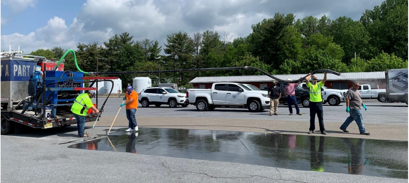
Figure 13 - Contractors demonstrate application process for high friction surface treatment at SHA service yard.
