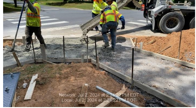
Figure 21 – New ramps being built at Good Hope Road and Briggs Chaney Road.
