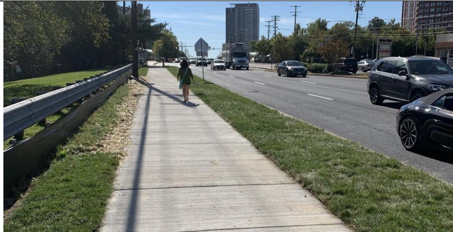
MCDOT widened the sidewalk and created a grass buffer between the sidewalk and roadway along Rockville Pike.
