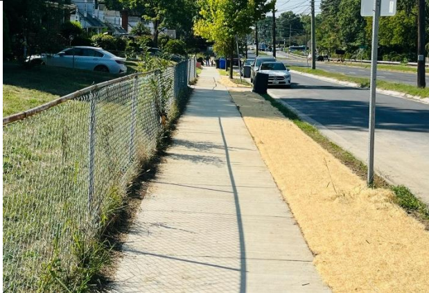
New sidewalk installed along New Hampshire Ave Service Road as part of high injury network project.
